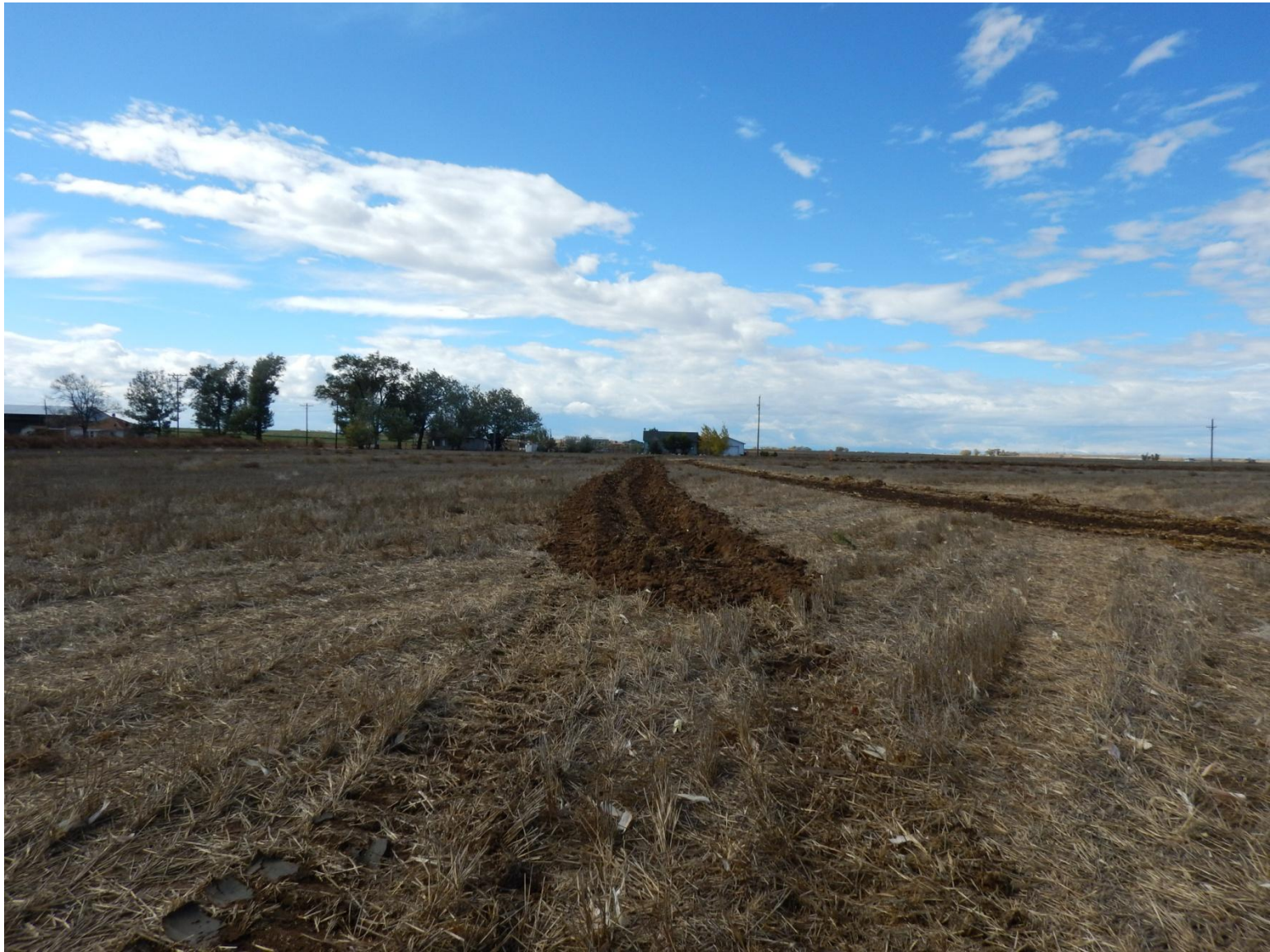
Photo 4: Photo taken from East side of location looking West. Stormwater control ditch center of photo.
