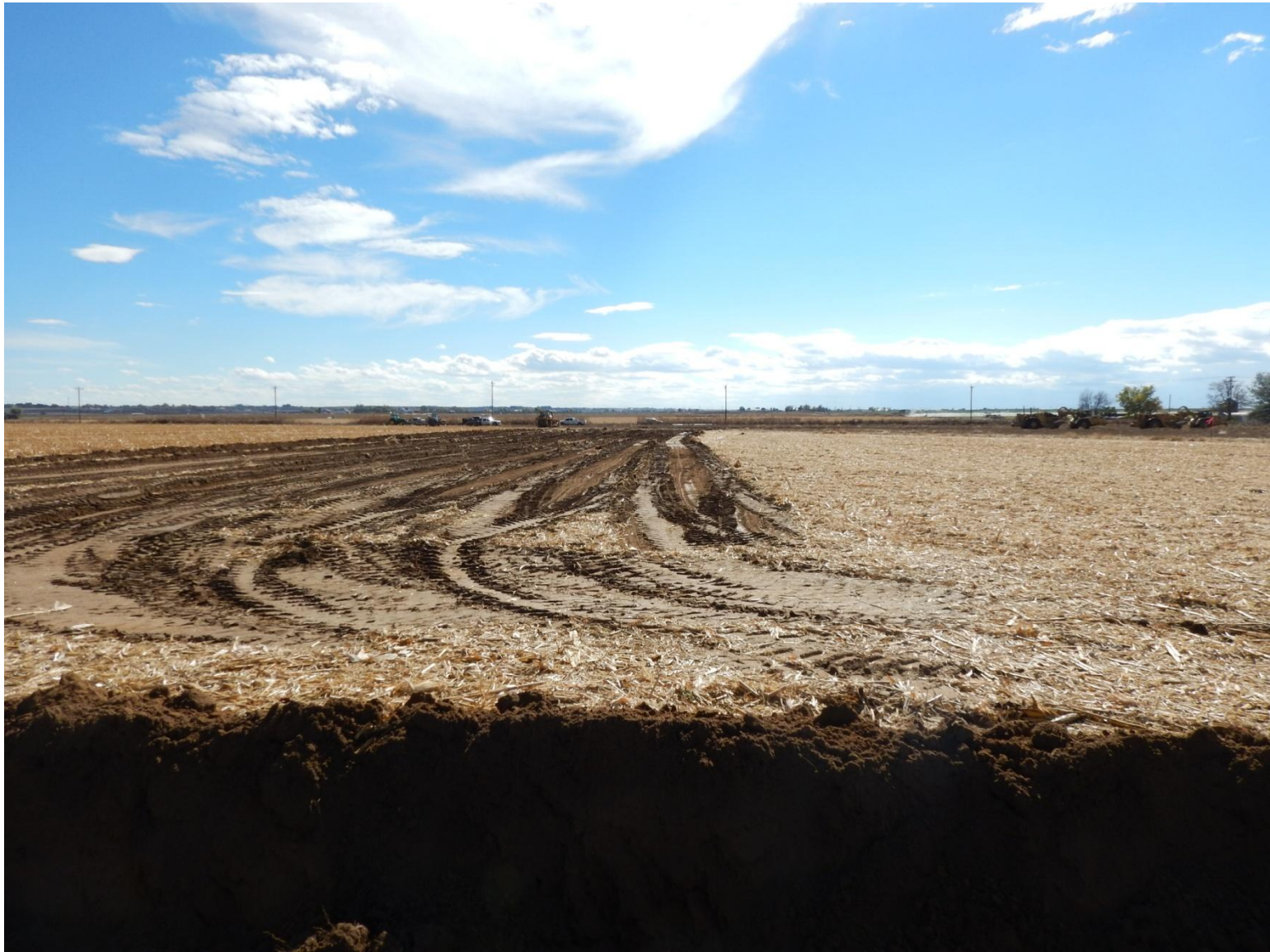
Photo 11: Photo taken from North side of location looking South. Topsoil removal in process.
