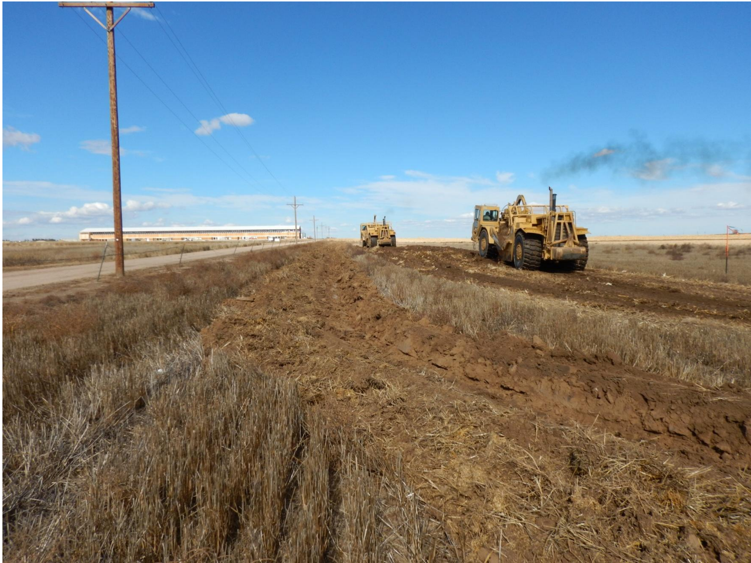
Photo 7: Photo taken from West side of location looking North. Note scrapers depositing topsoil. Stormwater control ditch center.
