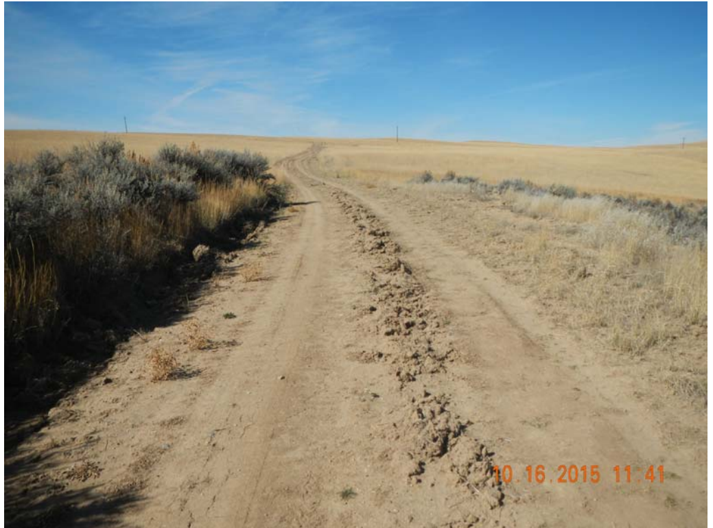
Rough and rutted road.
