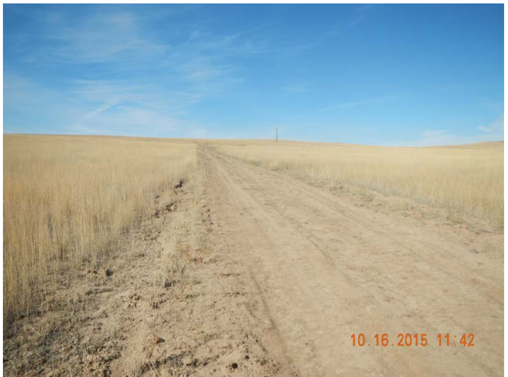
Rough and rutted road.
