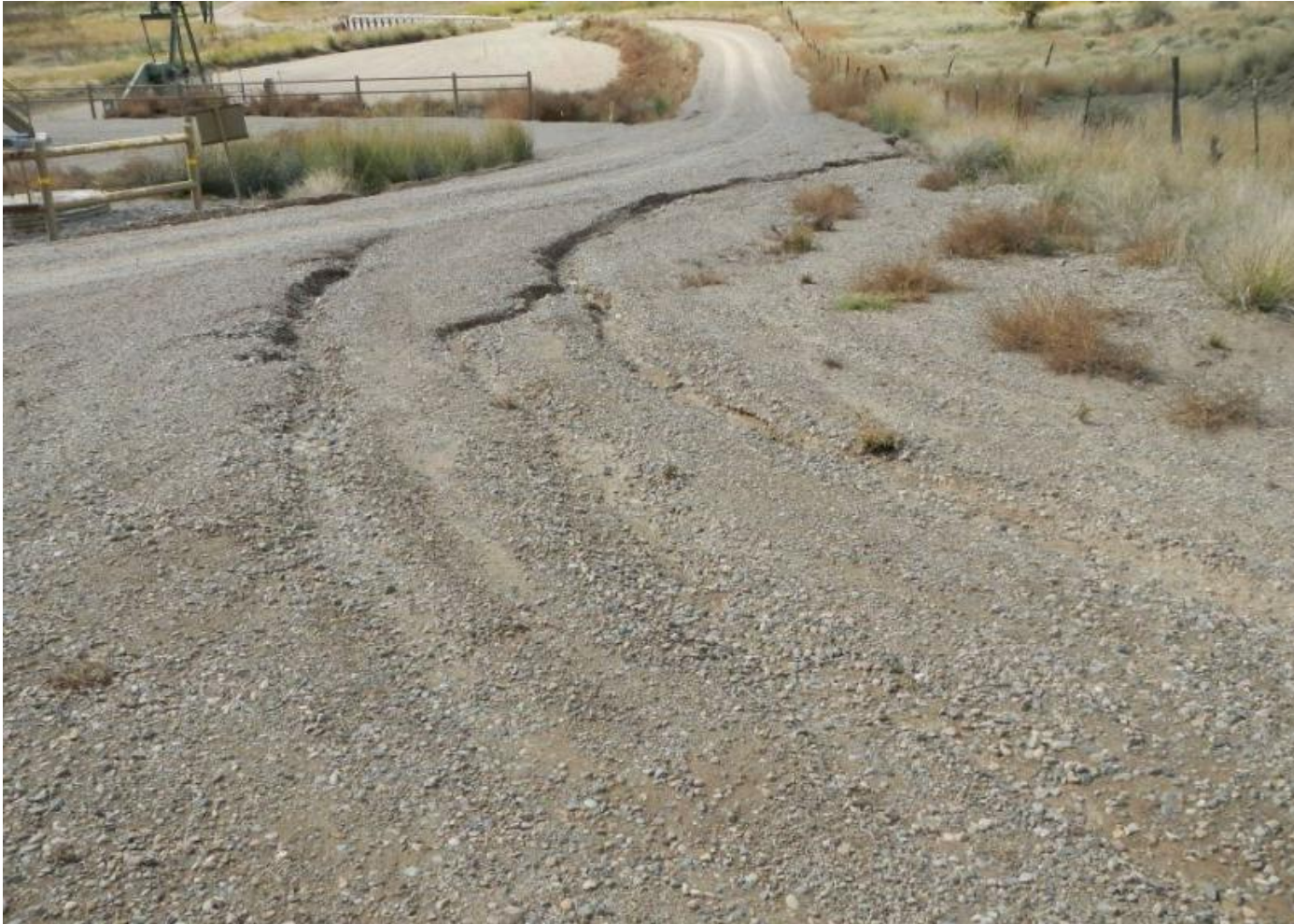
Photo 8. View of erosion along access road facing westward from beginning of access road. It appears concentrated stormwater flows over and erodes the road surface and continues down-slope.
