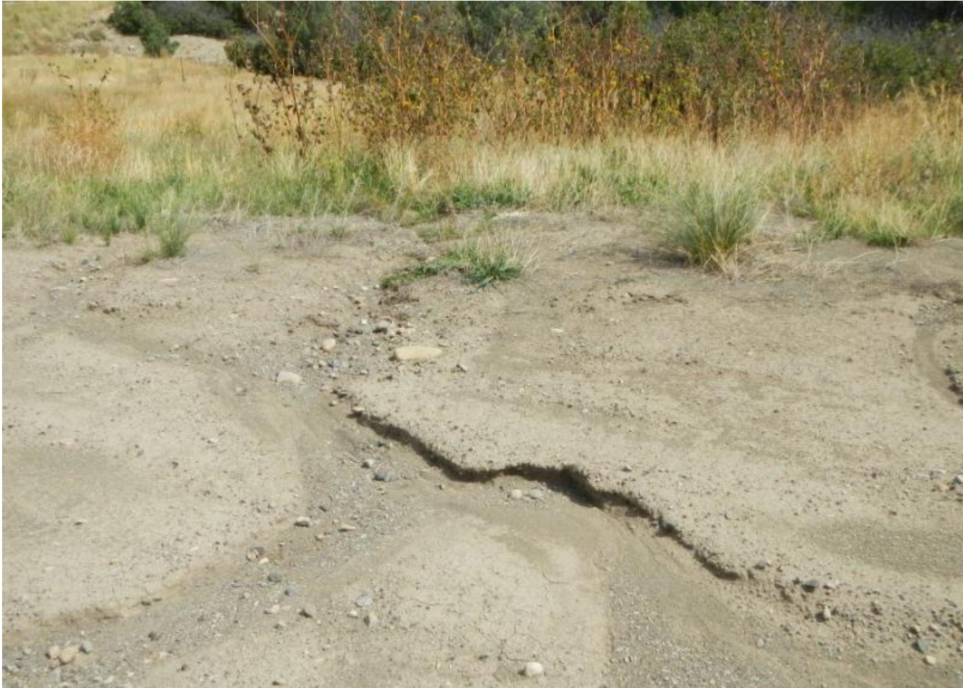
Photo 5. View of eastern edge of working area where concentrated stormwater flows exit the well pad.
