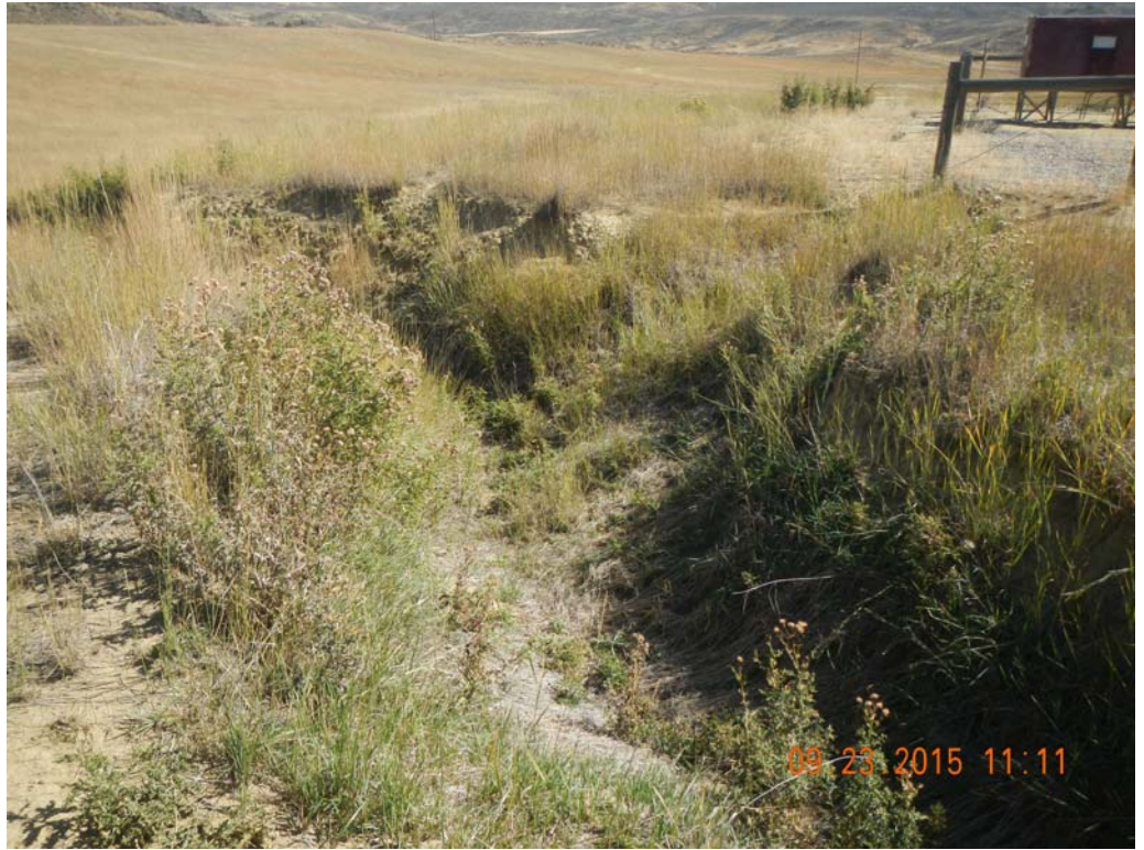
Erosion gully leaving location on north side. Noxious weeds visible on sides of gully.
