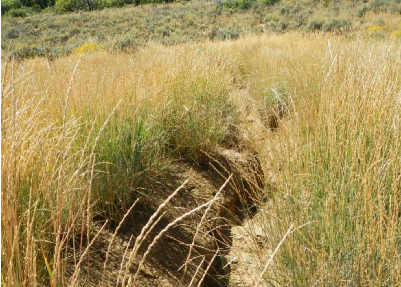
Photo 1. View of approximately 2 foot wide and deep erosional channel in western portion of project area.
