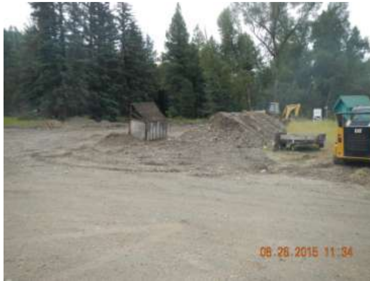
Hay Barn Construction – Located southeast of current shop area. No visual evidence of impacted material in excavation.
