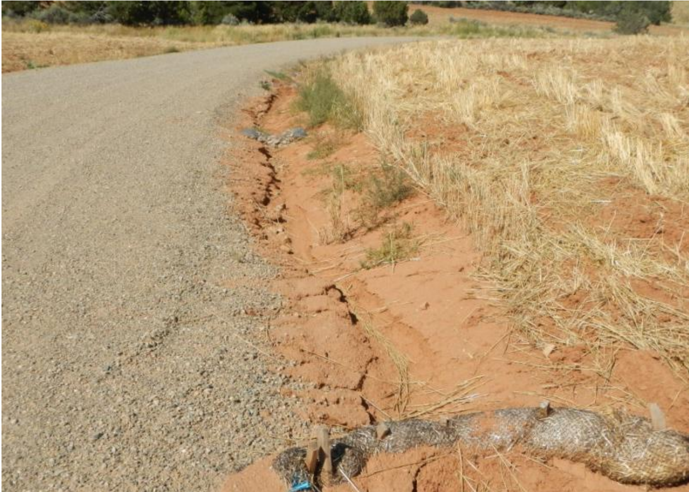
Photo 4. View of erosion occurring along eastern edge of the access road. Incision from high energy flows is observable between wattles and sediment accumulation above and around wattles is apparent in foreground.
