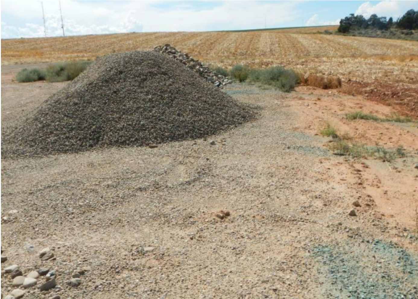
Photo 3. View northern portion of project area with stockpiled construction material facing westward from northeastern corner.
