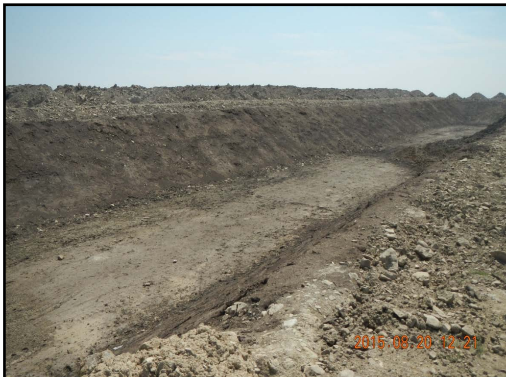
Pit in process of closure. Liner has been removed. No staining was observed at the bottom or on the walls.
