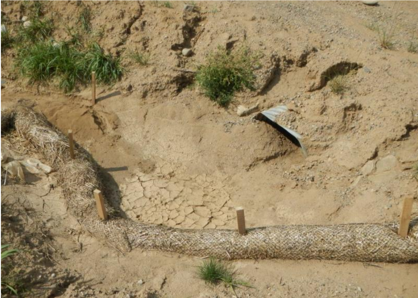
Photo 1. View of sediment filled silt trap and wattle at culvert near well pad entrance. This area needs stabilization and maintenance.
