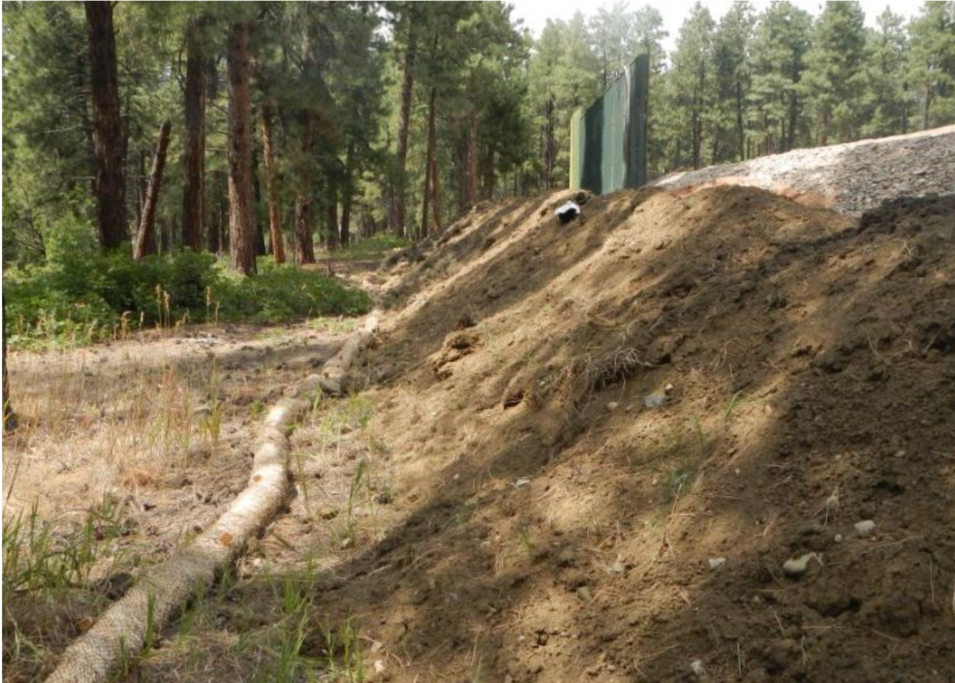
Photo 1. View of western edge of project area from southwestern corner facing northward. Perimeter wattle and soil stockpile in place.
