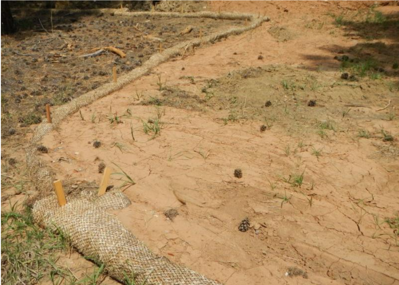
Photo 3. View of wattles on eastern edge of project area that need maintenance.
