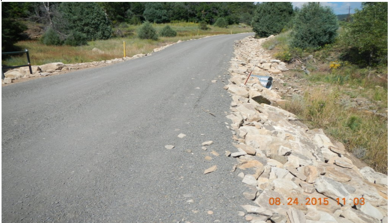
photo 2: Main access road traveling northwest towards the location. Road repairs have recently been performed.
