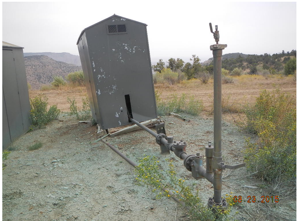
Disconnected meter house.
