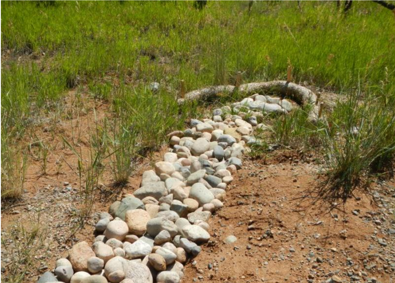
Photo 3. View of stormwater BMP within eastern portion of project area that appears to be functioning properly.
