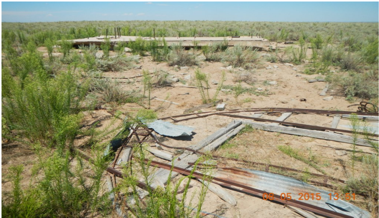
photo 2: Various metal debris and concrete slab left at the location.
