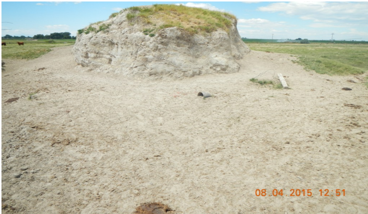
photo 10: Dirt mound has not been recontoured and is susceptible to erosion. Debris found along the base of pile.
