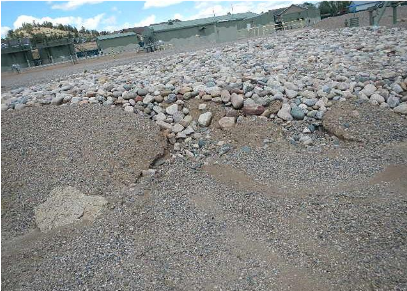
Photo 7. View of stormwater erosion from concentrated flows over the southwestern corner of well pad.
