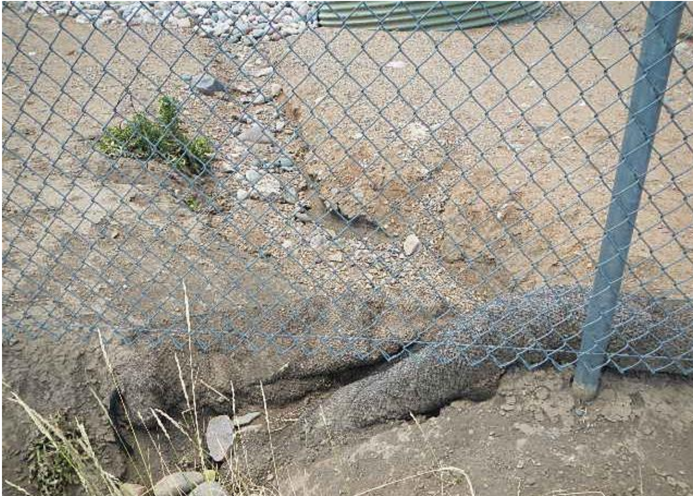
Photo 5. View of failed straw wattles in southern portion of project area.
