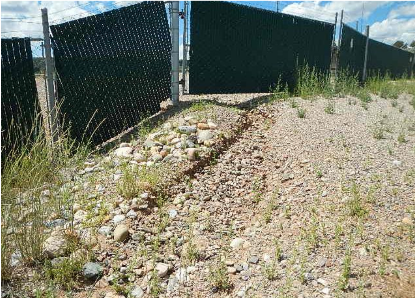
Photo 1. View of erosional channel flowing from well pad entrance. Dimensions are approximately 2 to 3 feet wide and 6 to 12 inches deep.
