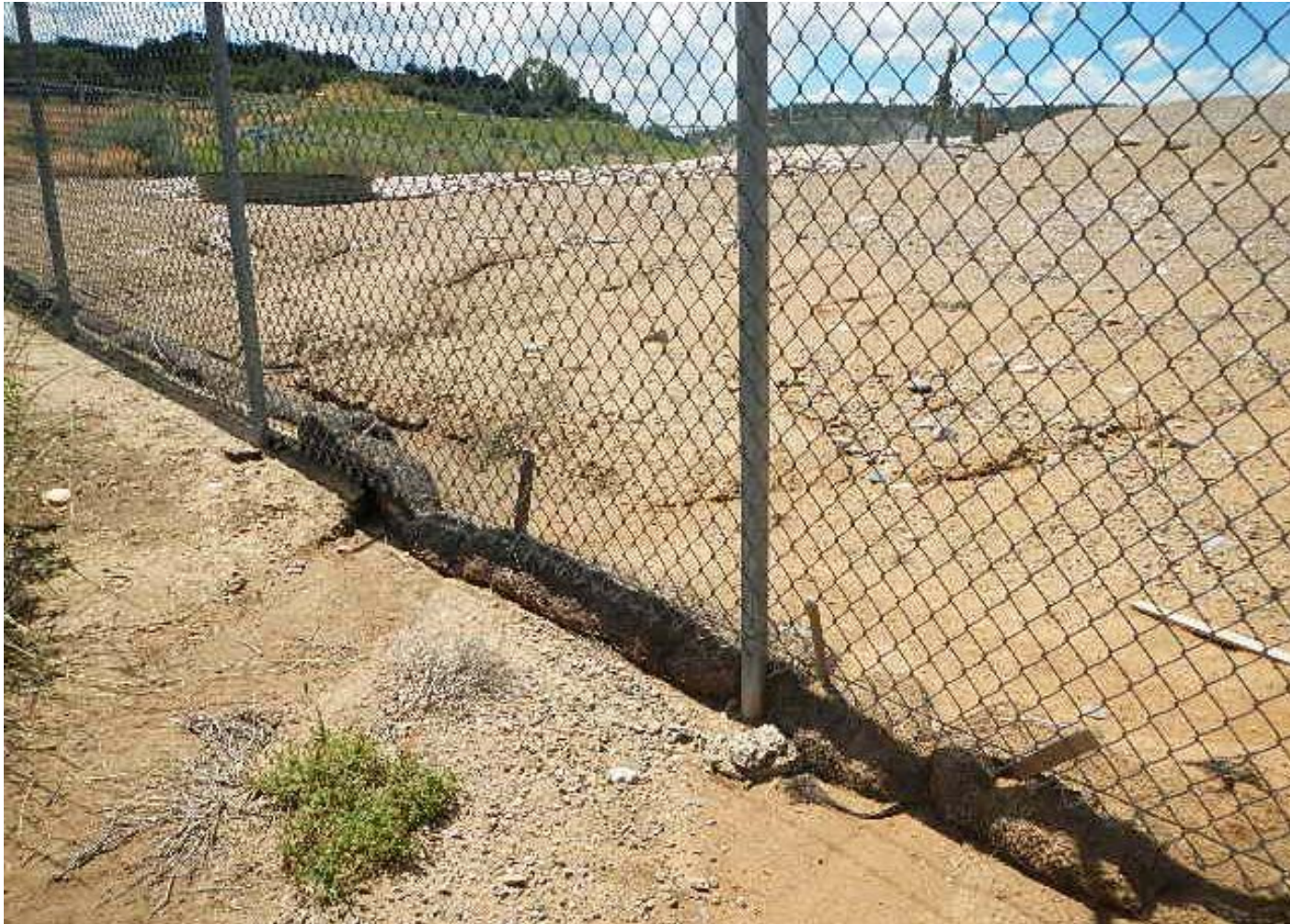
Photo 3. View of erosional channels flowing off of southern portion of project area.
