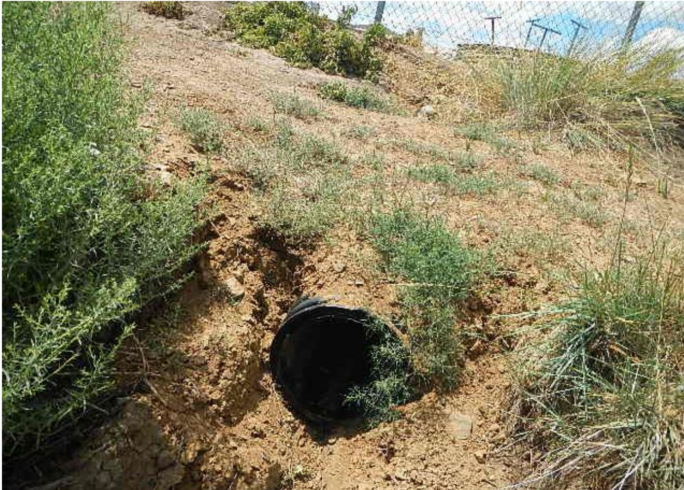
Photo 6. View of culvert that is not stabilized in southern portion of project area.
