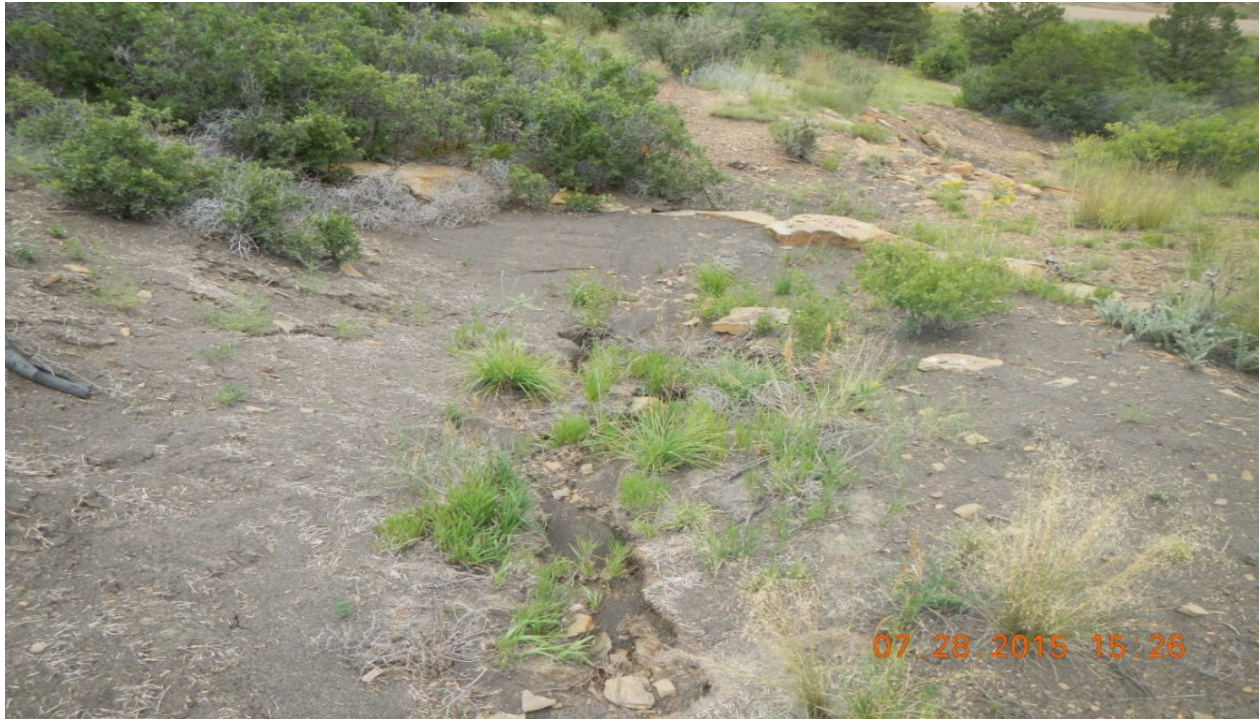
photo 9: Southeast side of the location has signs of erosion and sediment trap is filled with sediment.
