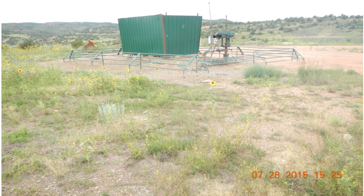
photo 8: Facing northwest towards the equipment.
