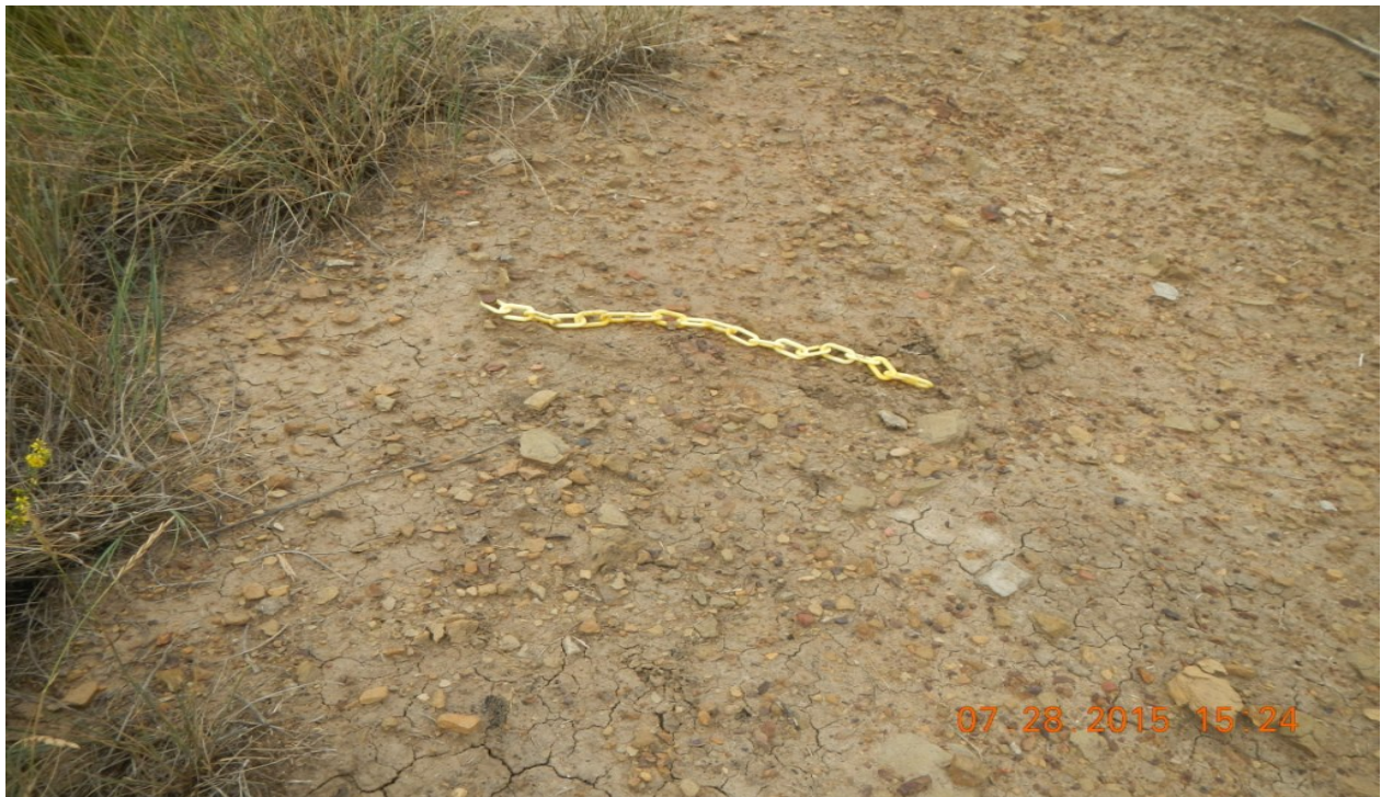
photo 4: Chain indicating 2 ft. freeboard is laying on a flat surface and does not appear to be installed correctly.
