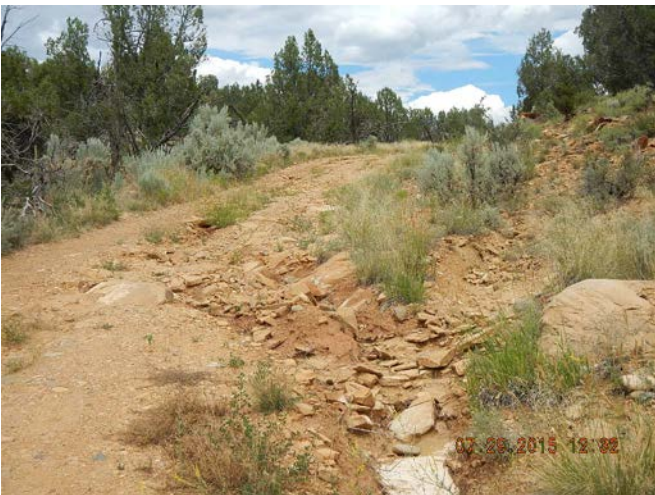
Stormwater damage on well site access road; Stormwater channel in access road.
