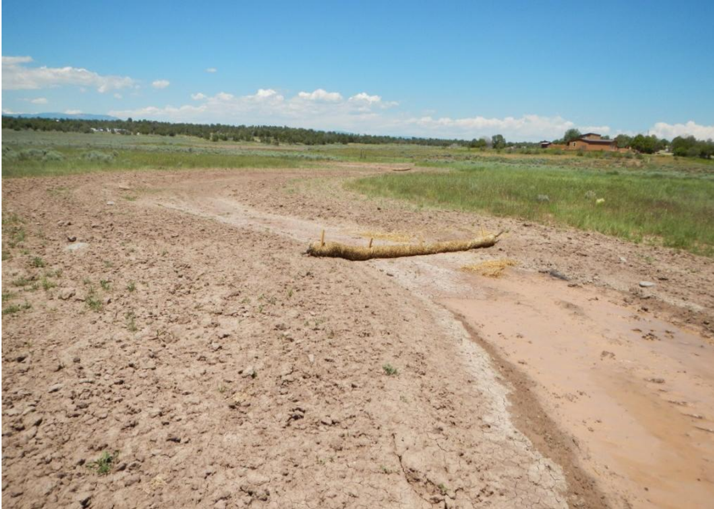
Photo 3. View of swale contoured into project area with straw wattles. From eastern edge of well pad facing northeastward.
