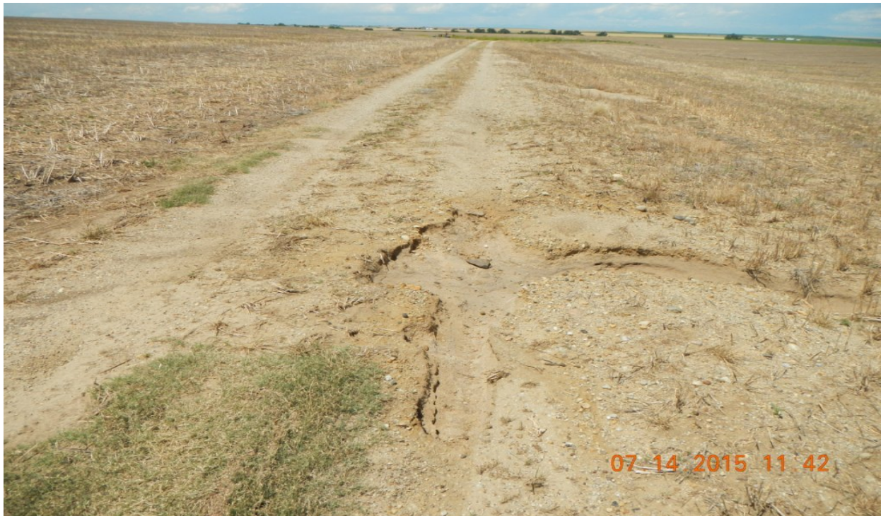
photo 5: Erosion is occurring along the access road traveling west towards the location.
