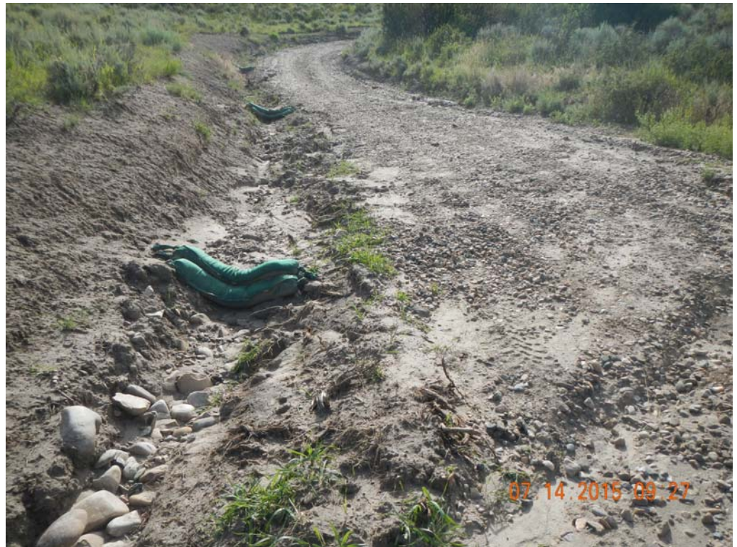
Full sediment traps causing erosion on access road.
