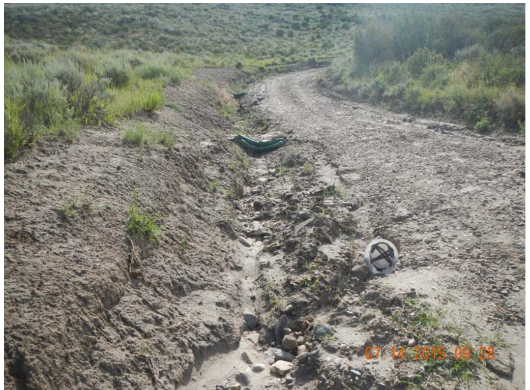
Full sediment traps with erosion. (Hard hat shown for scale of gullies.)
