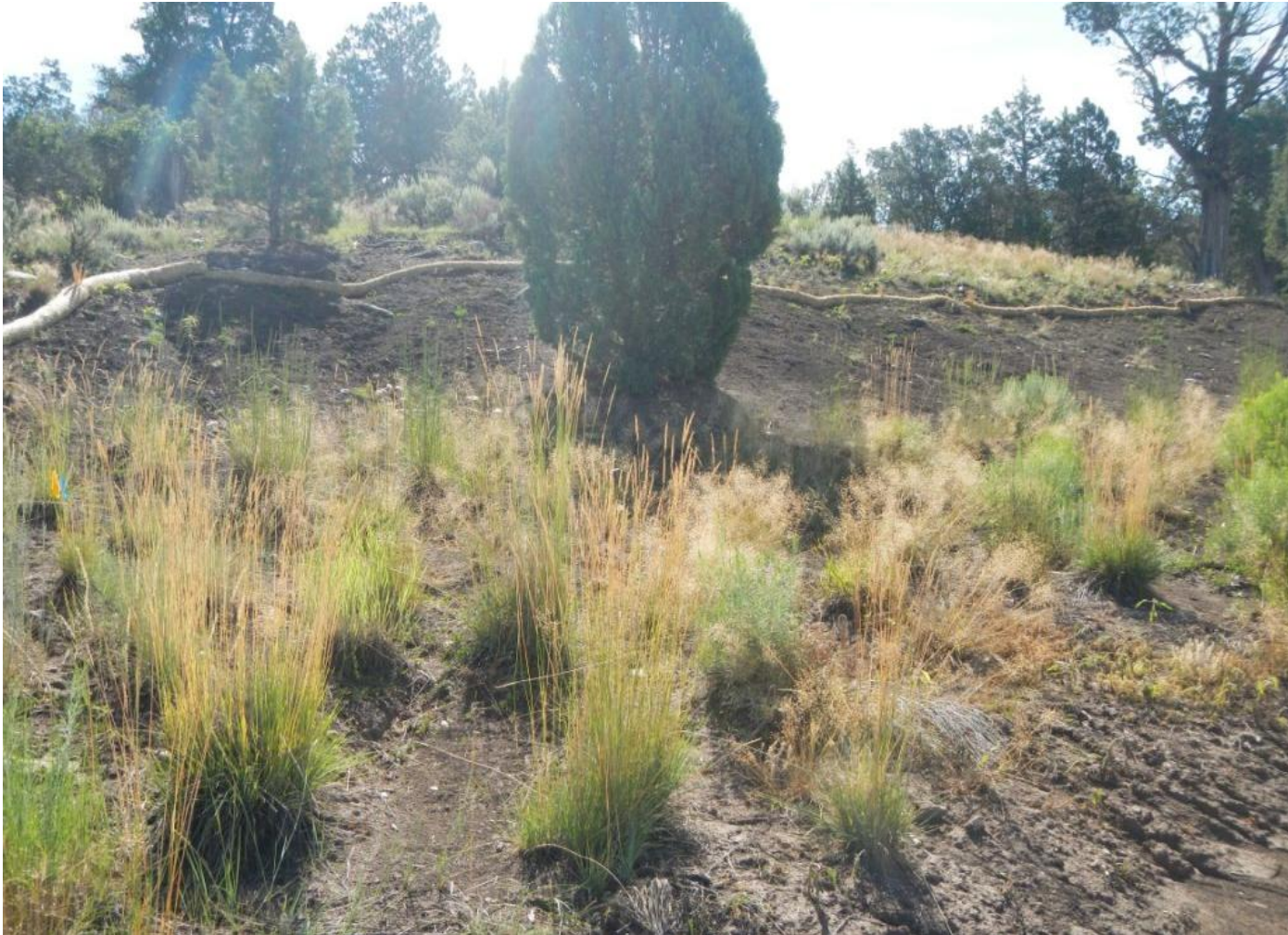
Photo 4. View of newly installed straw wattle near the top of the eastern cut-slope.
