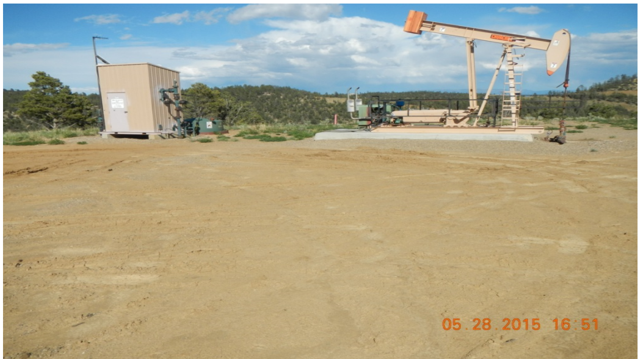
photo 2: Facing west towards the production equipment.
