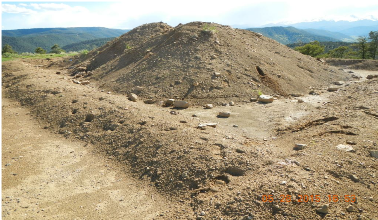
photo 6: Topsoil pile is not protected from erosion and should be stabilized with vegetation.
