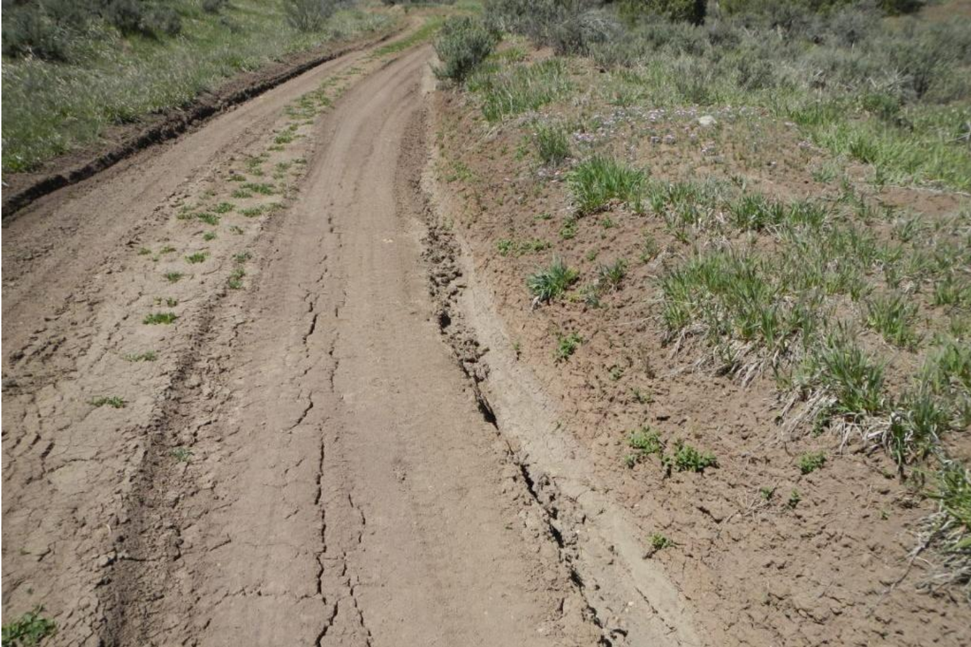
Photo 8. View of stormwater erosion channels that flow along both sides of access road.
