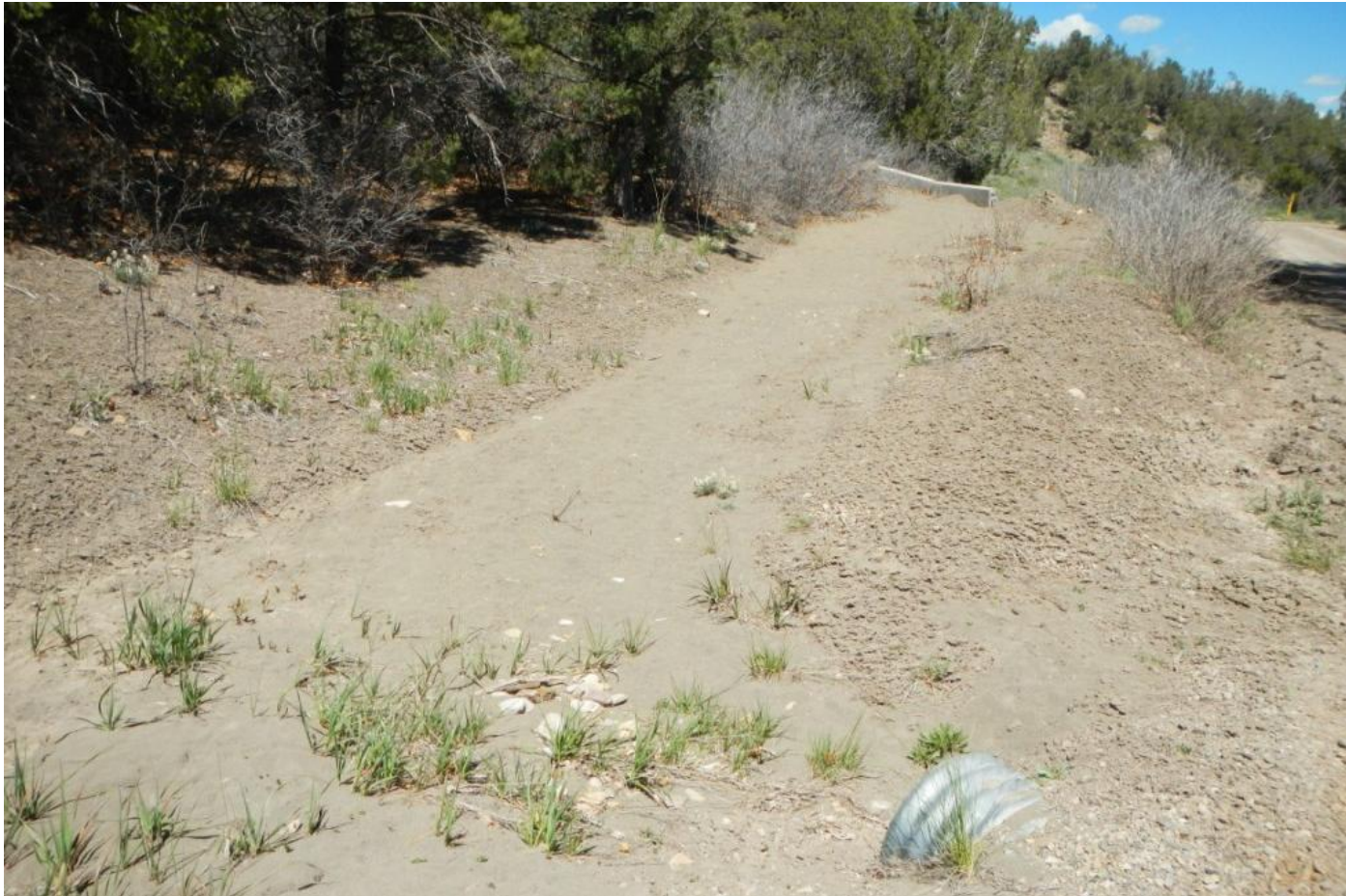
Photo 6. View of sediment filled drainage and culvert on access road.
