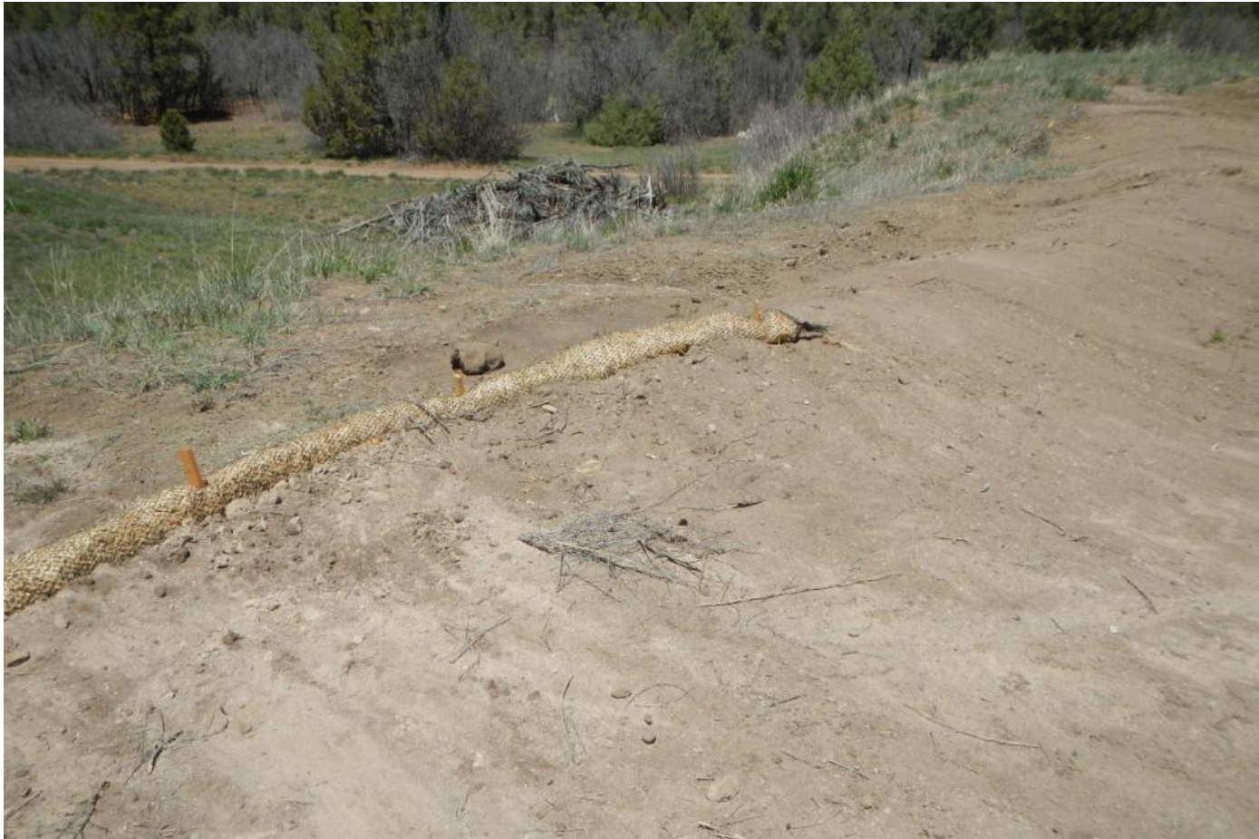
Photo 3. View of newly installed/maintained stormwater BMP along western edge of project area.
