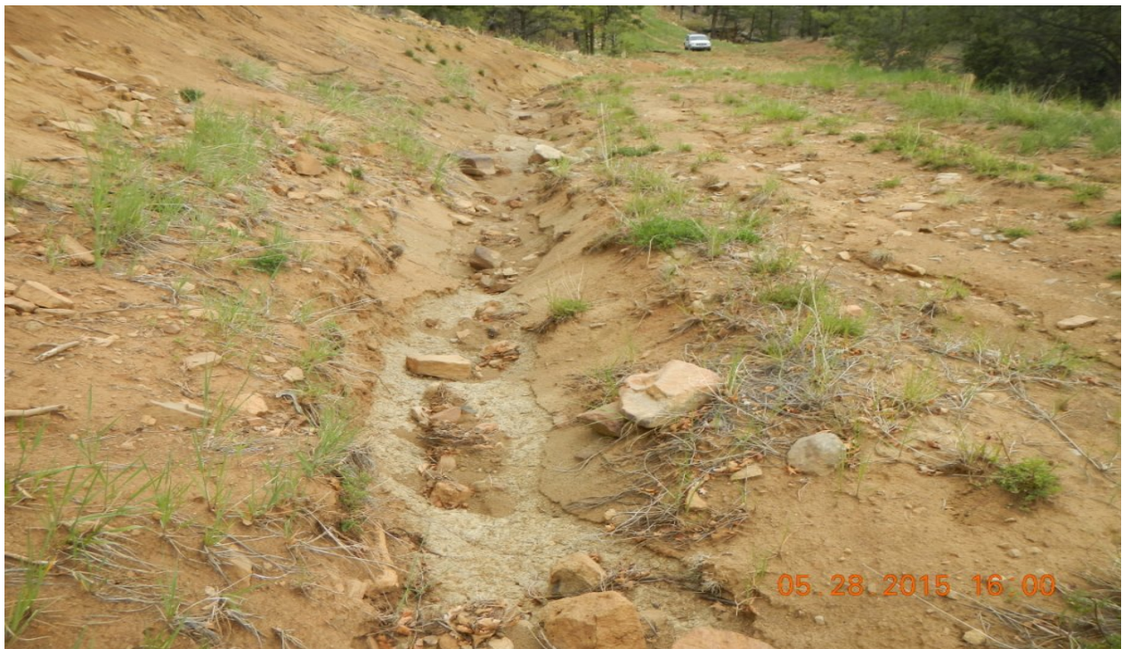
photo 4: Facing east. Erosion channels running down the access road.
