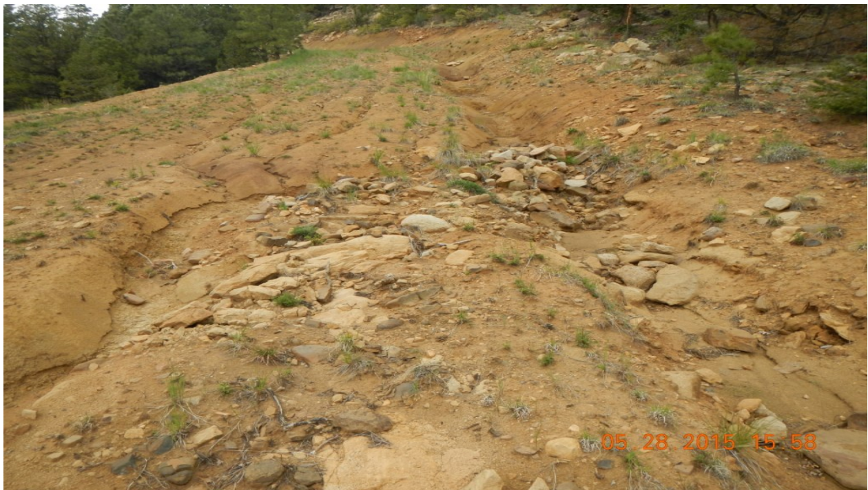
photo 2: Erosion rills/channels have formed transporting sediment and eroding the access road.
