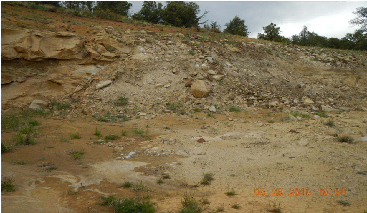
photo 10: North side of the location. Unstable cut with material falling onto the pad.
