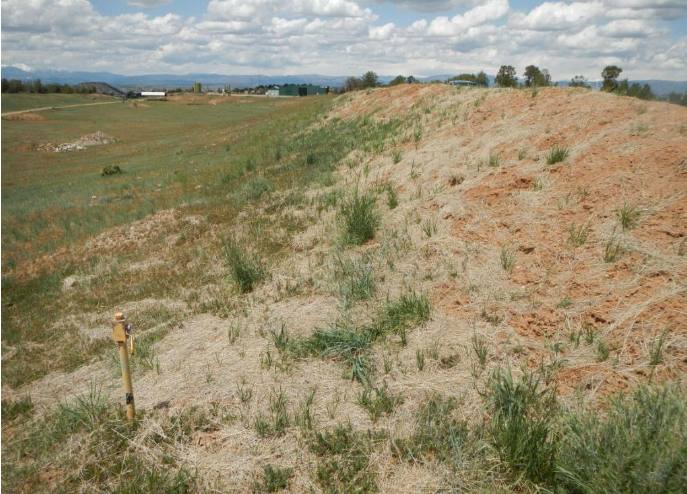
Photo 4. View of western portion of project area. Straw mulch appears to be helping to stabilize the slopes.
