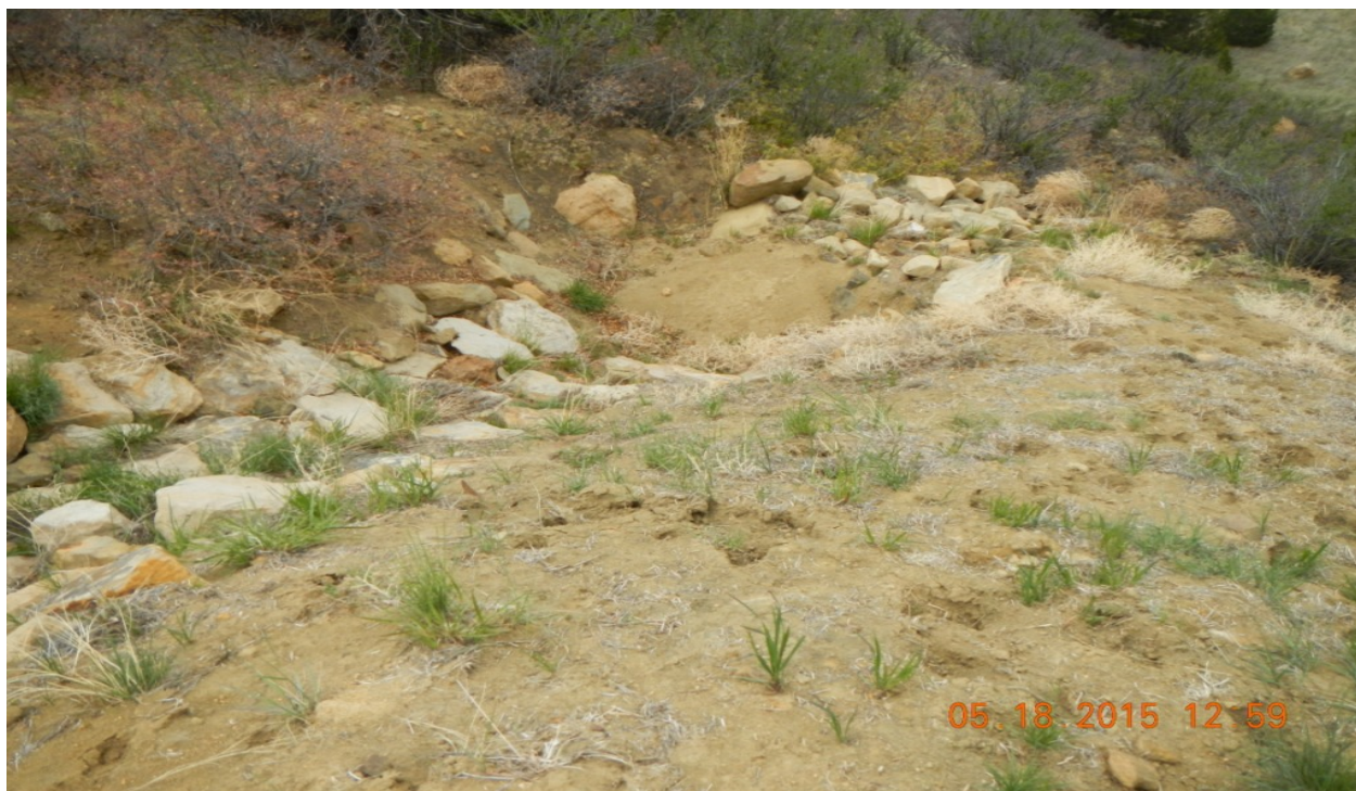
photo 4: Sediment trap at the east side of the location is filled with sediment.
