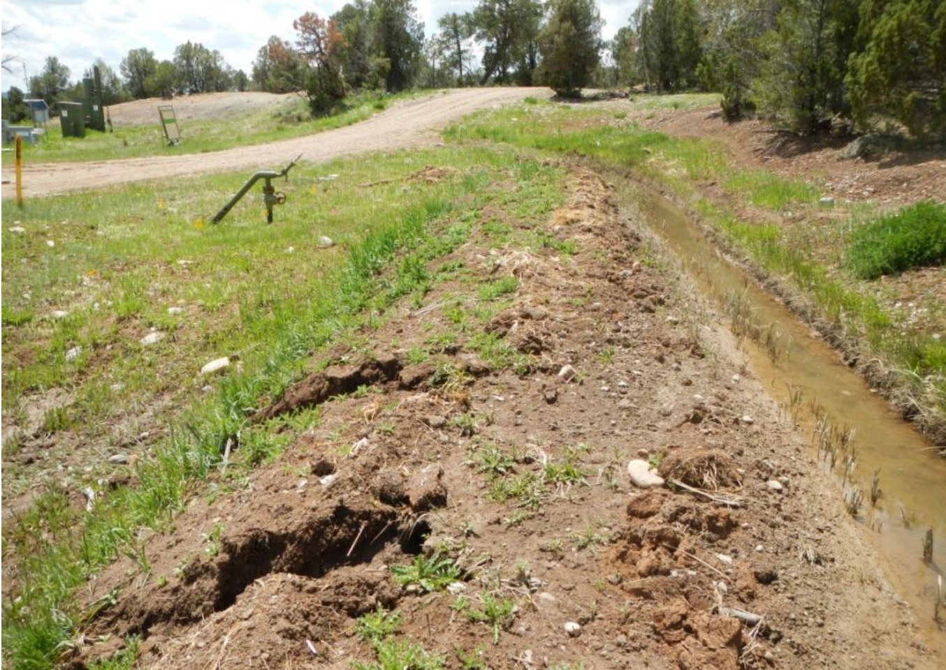
Photo 3. View of erosion where it appears ditch bank has breached along western edge of project area.
