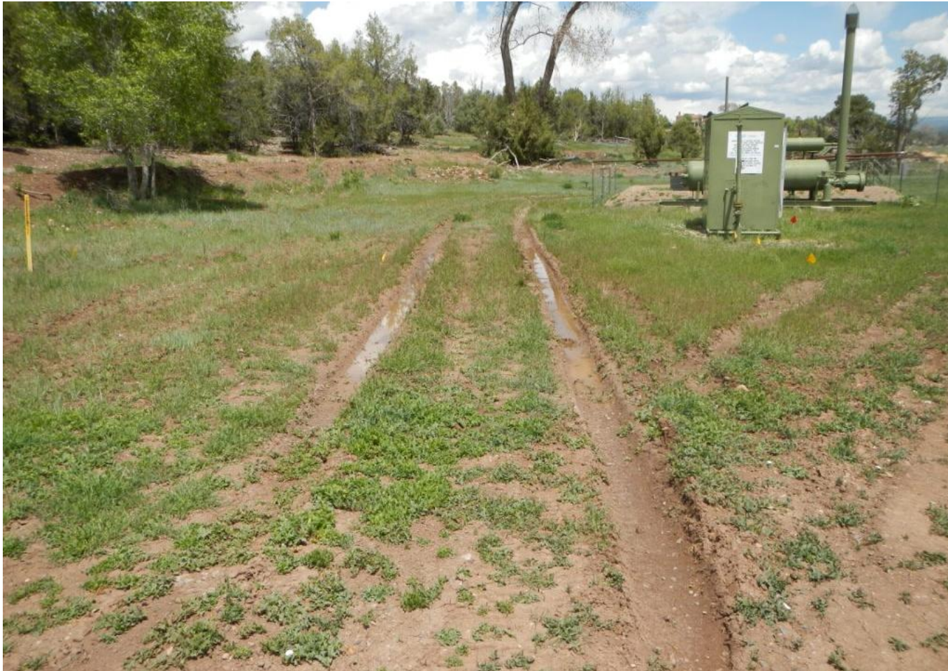
Photo 4. View of standing water in driving surface of well pad.
