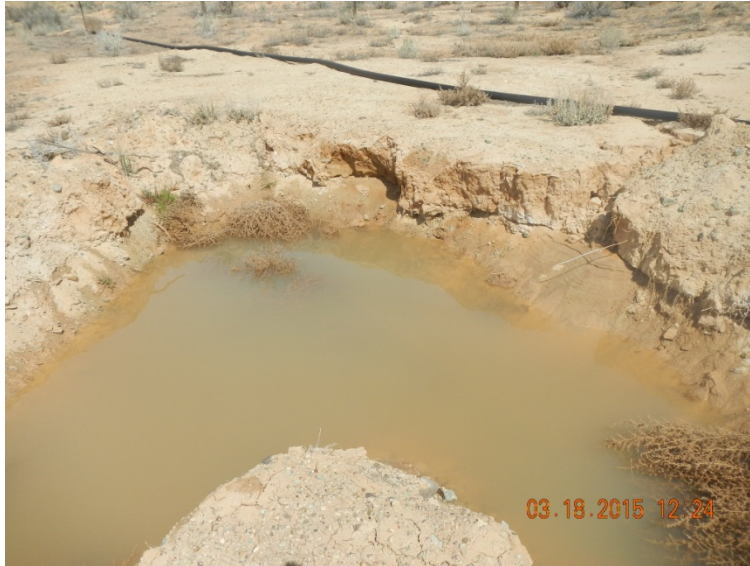
Open excavation from Spill #3 in East Fork McElmo Creek valley. Underground flow line can be seen in pool of standing water. No sheen or odor noted during this inspection. Replacement poly flow line can be seen behind excavation.
