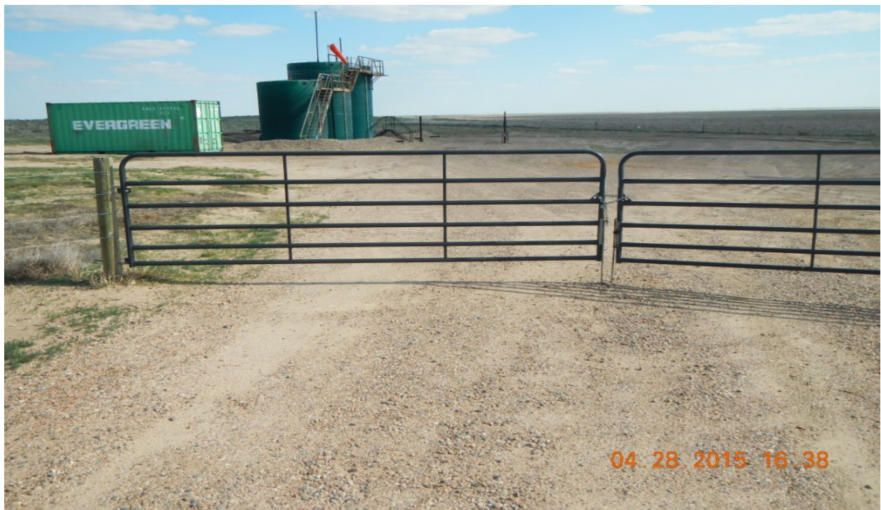
photo 2: Facing southeast towards the tank batteries and storage container.
