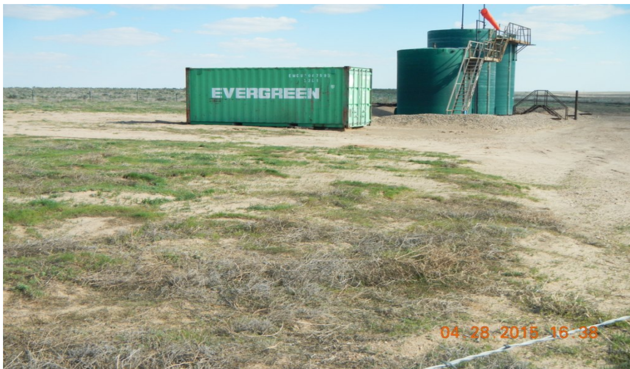
photo 3: Facing southeast towards the tank batteries and storage container.
