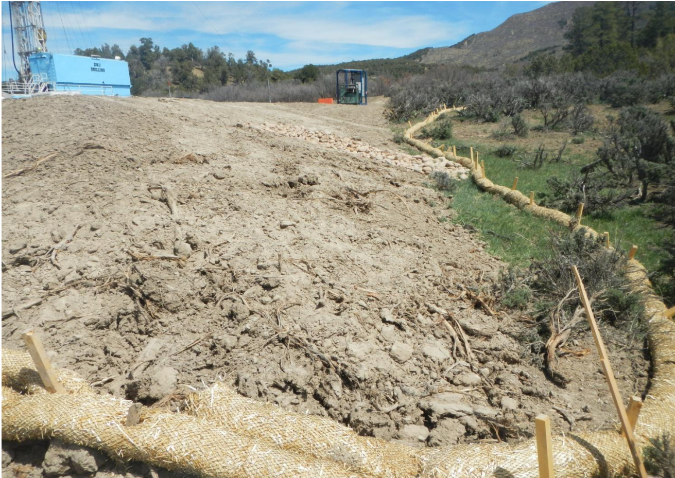
Photo 2. View of southern edge of project area from southwestern corner facing eastward. Straw wattles and cobble outlet can be seen.
