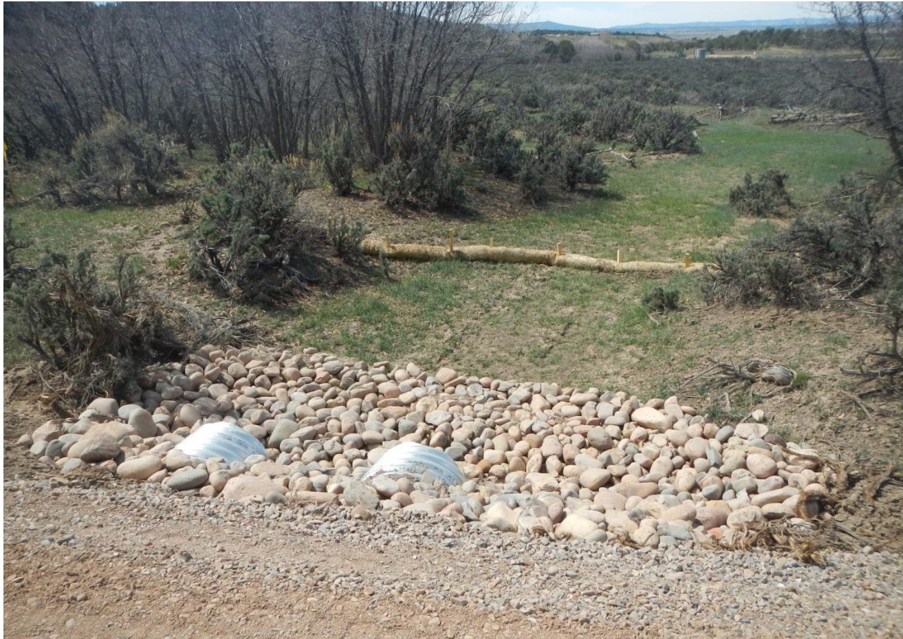
Photo 3. View of culvert outlet near entrance to well pad. Straw wattles and cobble armoring can be seen.
