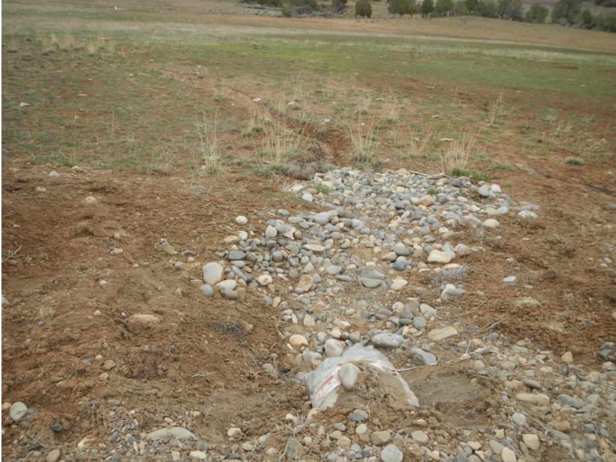
Photo 4. View of culvert outlet along access road where it appears cobble BMP may not be sufficient to de-energize concentrated flows that are diverted from the well pad.
