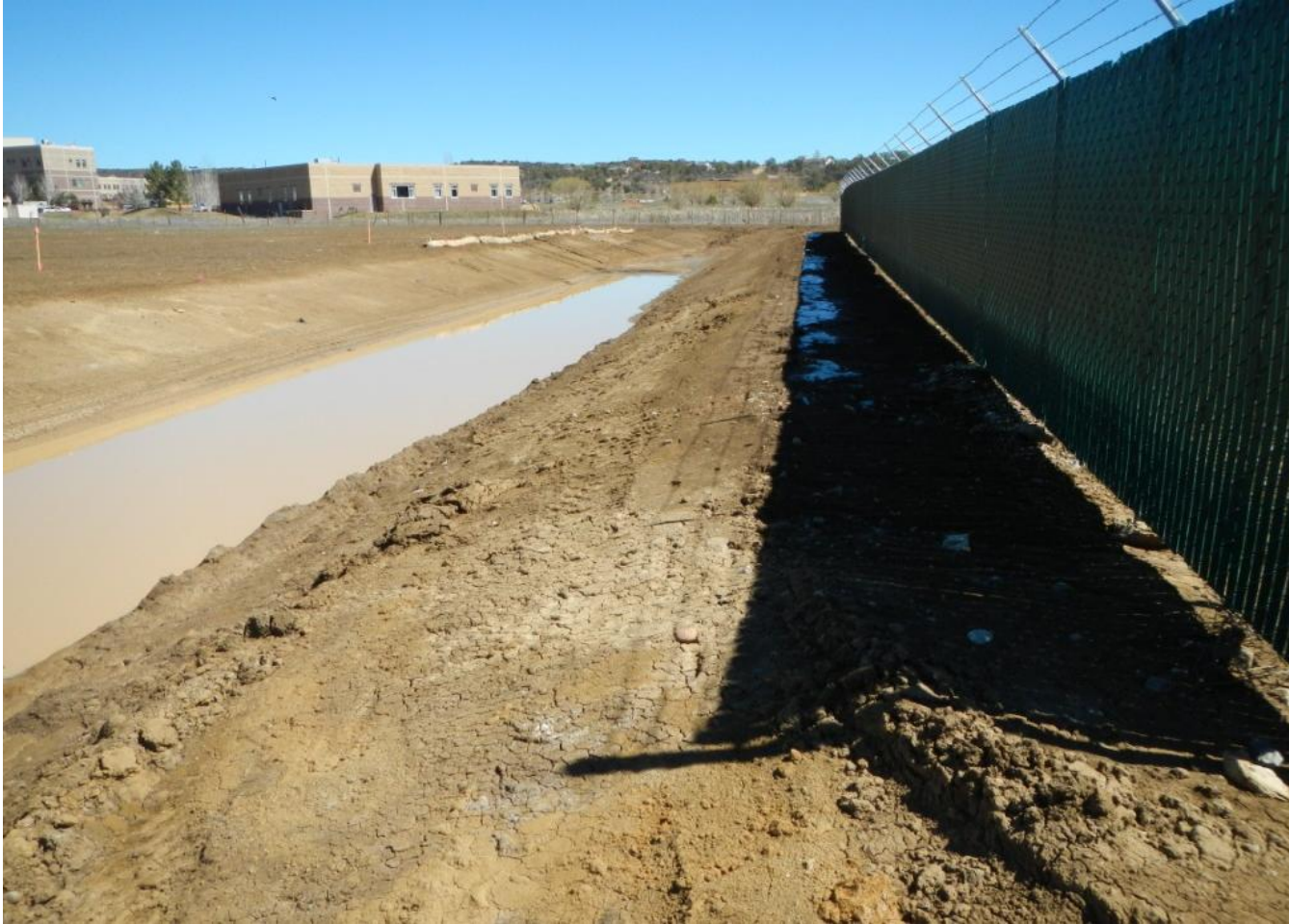
Photo 1. View of newly constructed canal along northern edge of project area from northwestern corner facing eastward.
