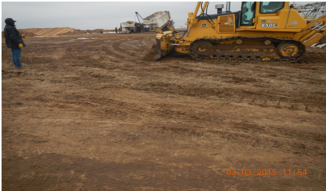
photo 15: Dozer pushing topsoil, leveling the pad. Top soil compacted and being mixed.
