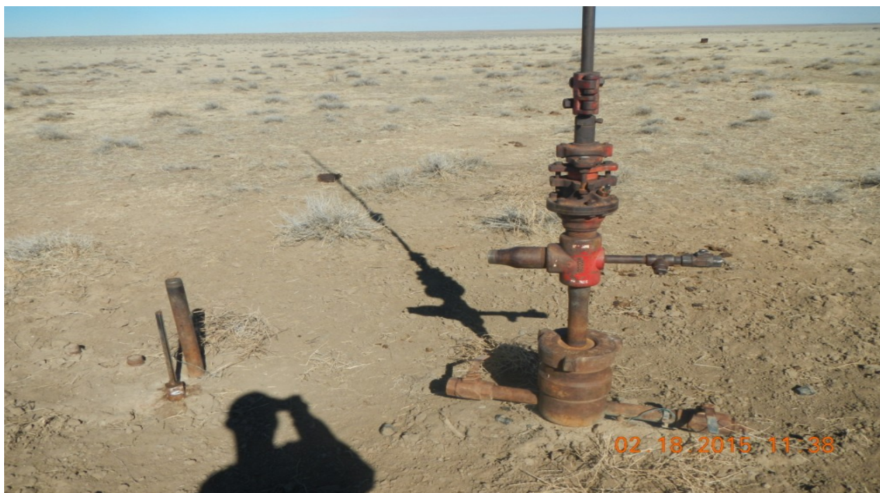
photo 2: Well head remains and pipe sticks out of ground. Lat/Long: 38.42055/-103.00909
