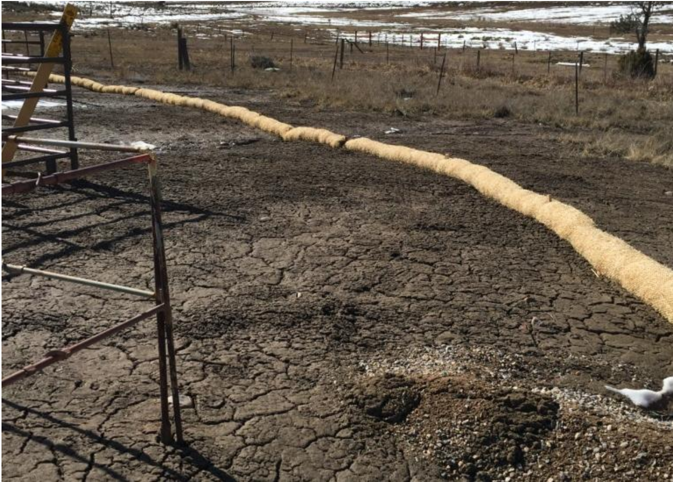
Photo 4. View of newly installed straw wattle placed along the western edge of the project area.
