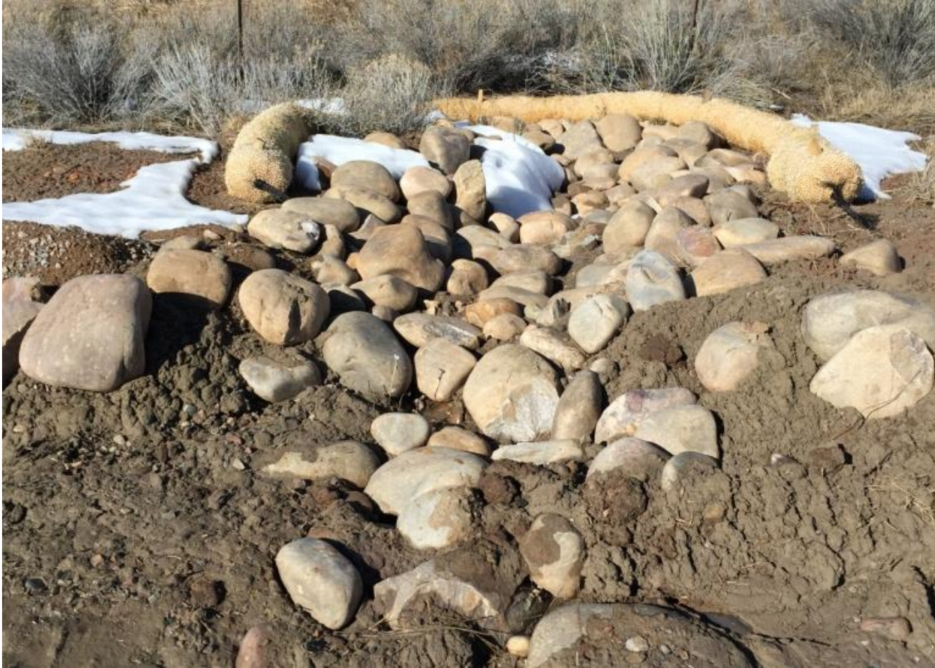
Photo 3. View of new cobble and straw wattle stormwater BMP where concentrated stormwater flows exit the northern portion of the project area.
