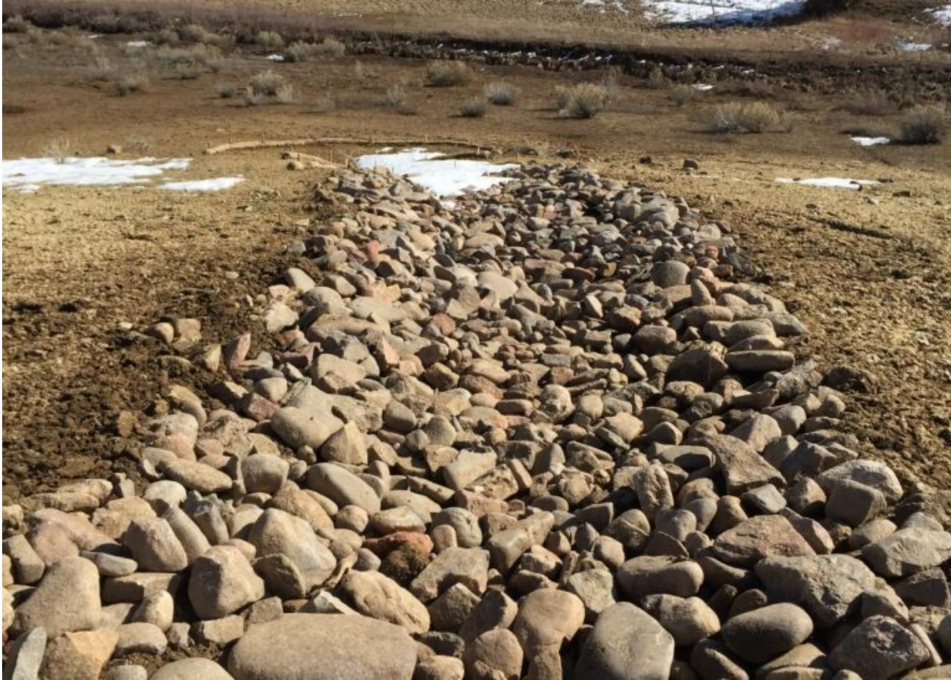
Photo 3. View of the bottom of a newly installed diversion channel, hydromulch, and straw wattles. Channel appears to be sufficient to de-energize and filter flows toward the irrigation canal shown in background.
