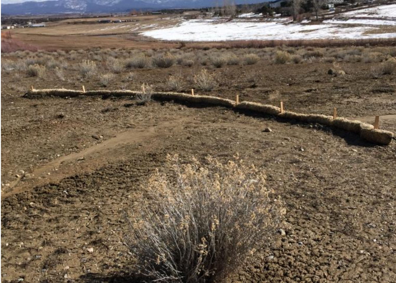
Photo 4. View of area in northeastern corner of project area where diverted stormwater flows from the northern edge of the well pad.
