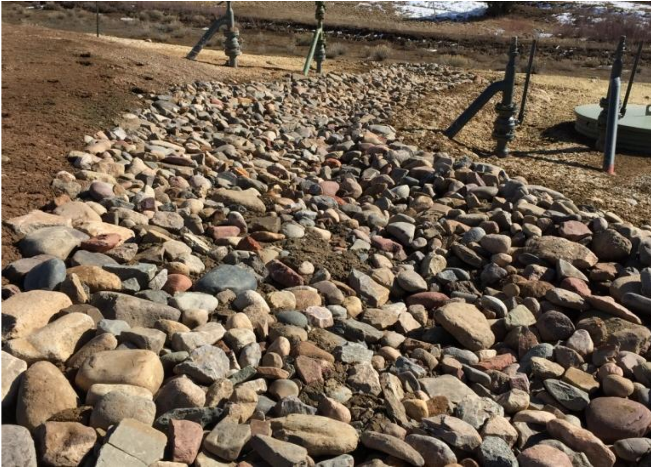
Photo 2. View of the top of a newly installed diversion channel in southeastern corner of project area.
