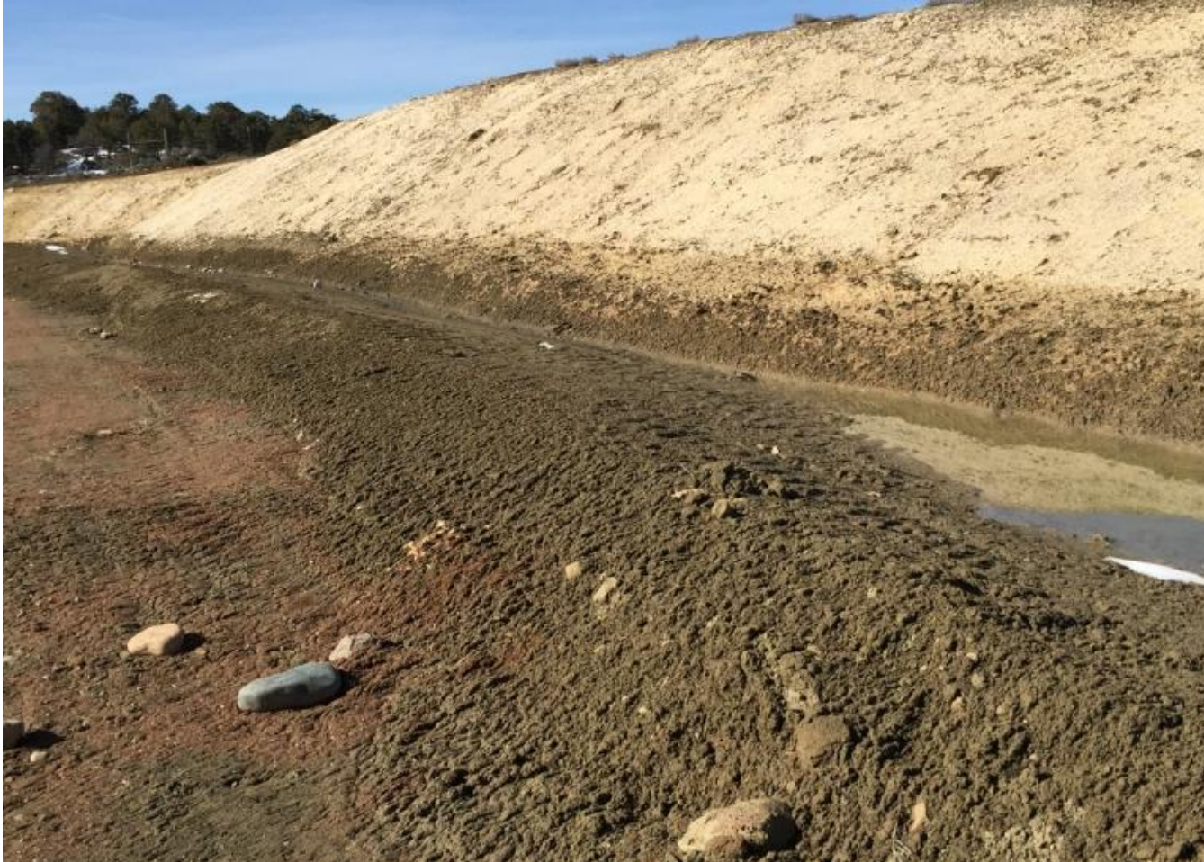
Photo 5. View of newly installed berm and hydromulch in northern and northwestern portions of the project area from northern edge facing westward.
