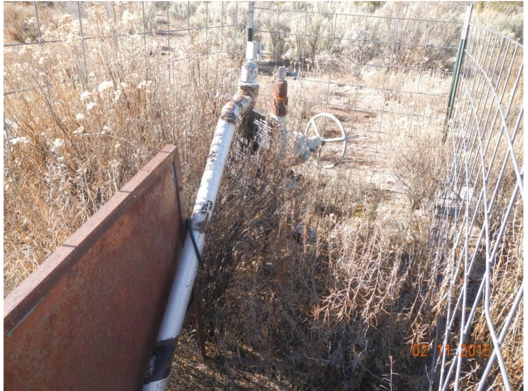
Weeds and vegetation around wellhead.
