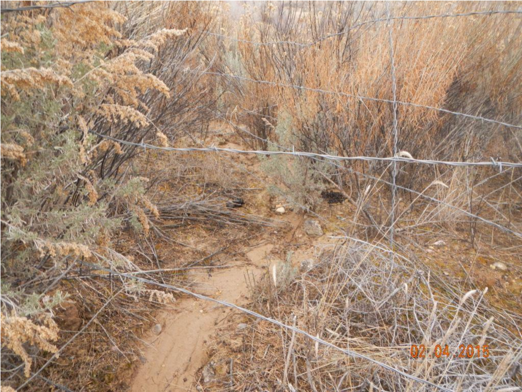
Road side erosion at entrance and sediment migration.
