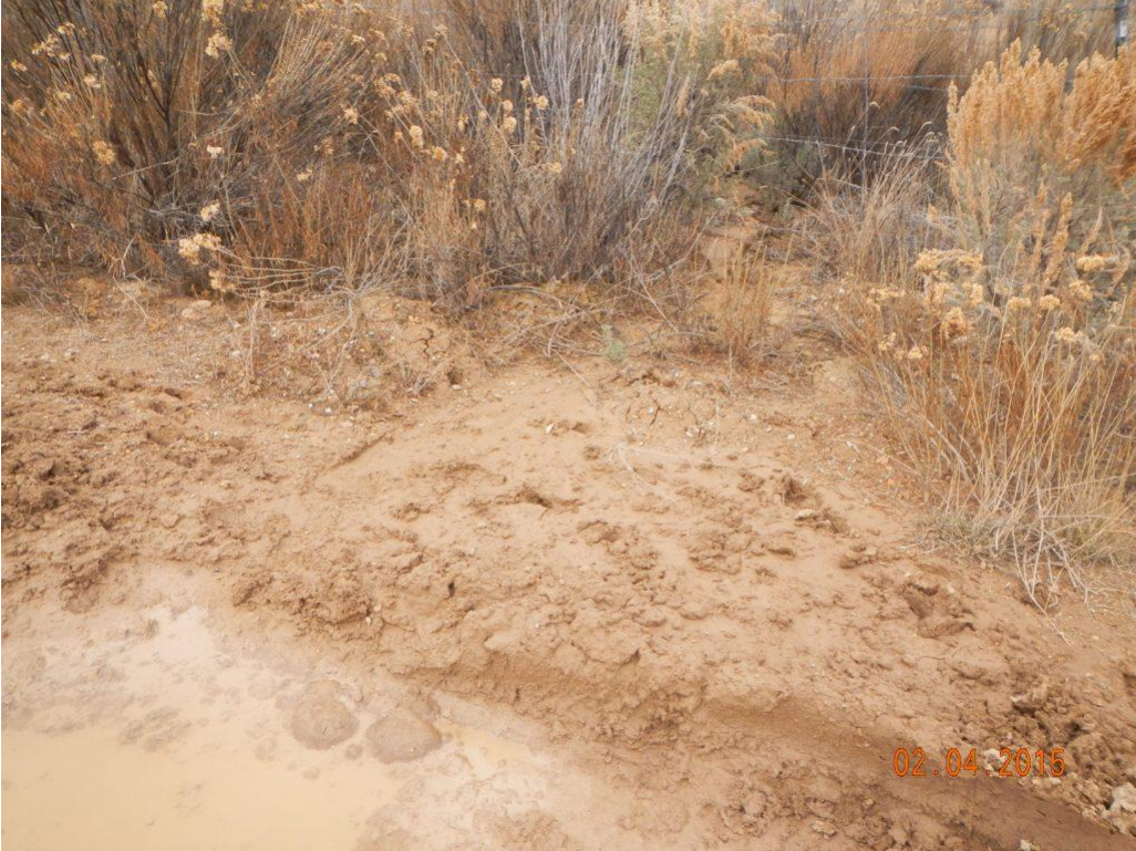
Road side erosion at entrance.
