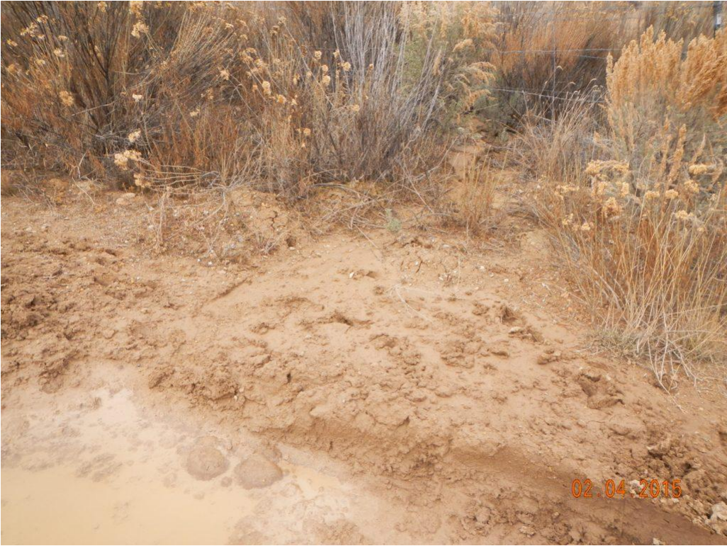
Road side erosion at entrance.
