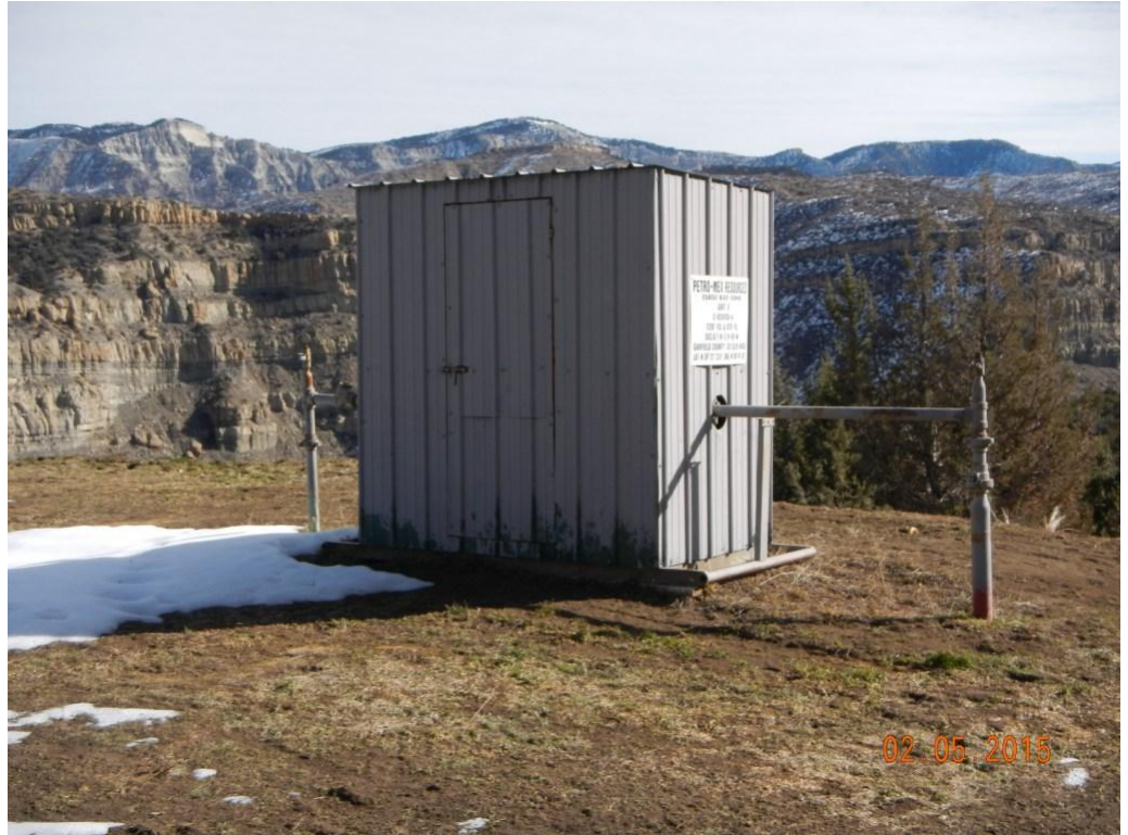
Gas meter on location.
