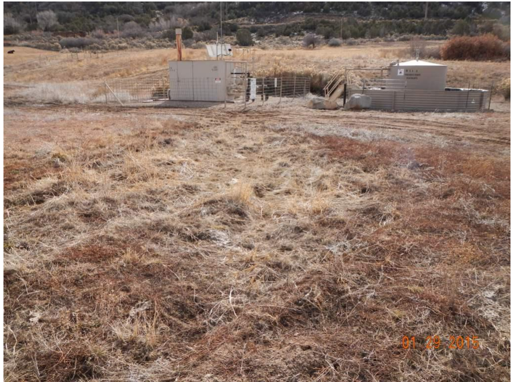
Subsidence between separator and wellhead over lines.
