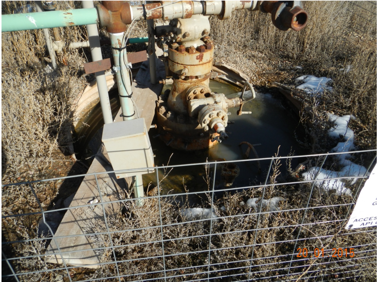
10. Well head cellar hole retaining water.
