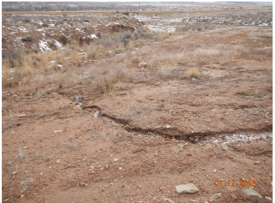
Erosion on SW side of location
