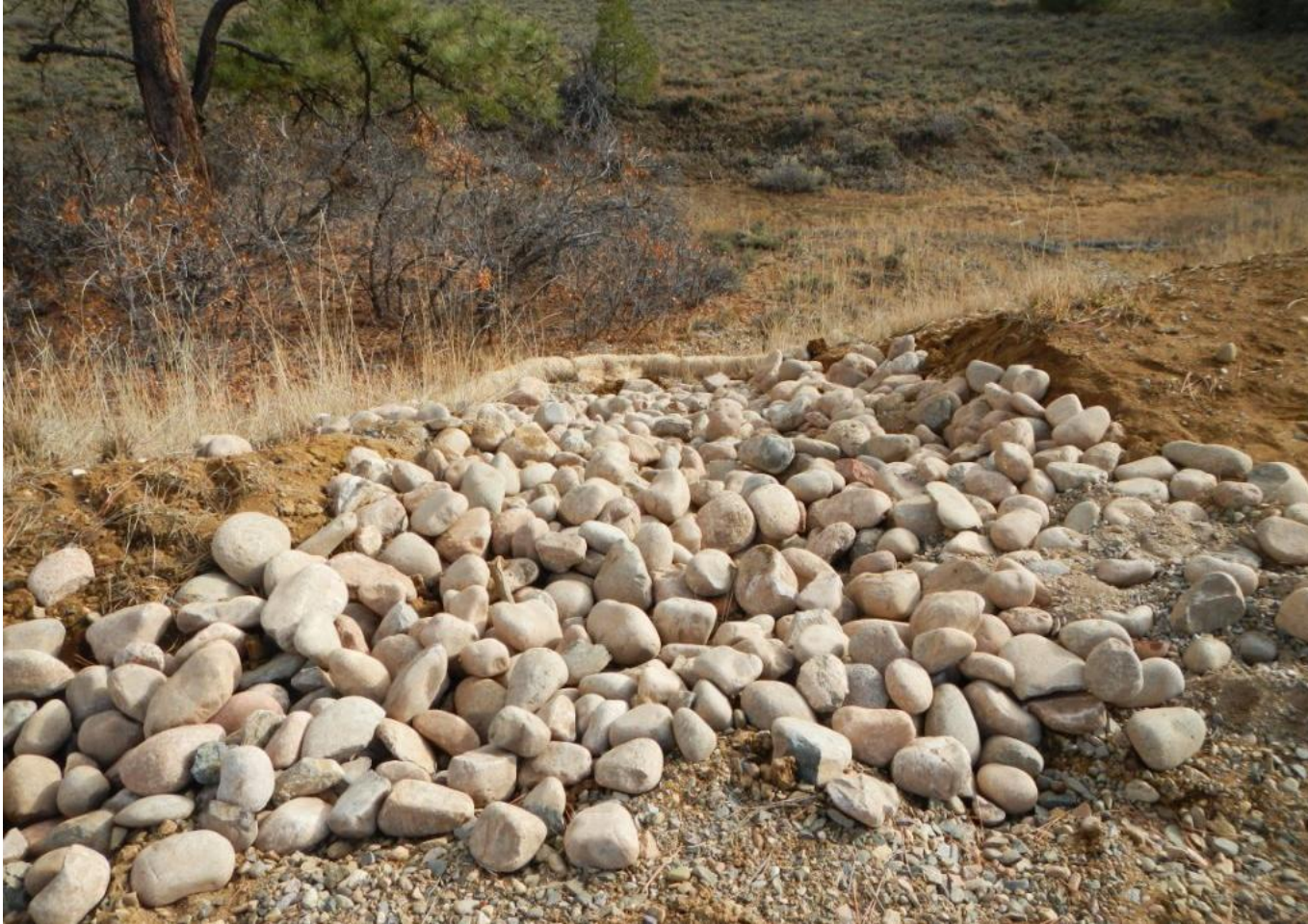
Photo 4. View of new BMP in eastern portion of project area with cobble in erosional gully and straw wattle placed below.
