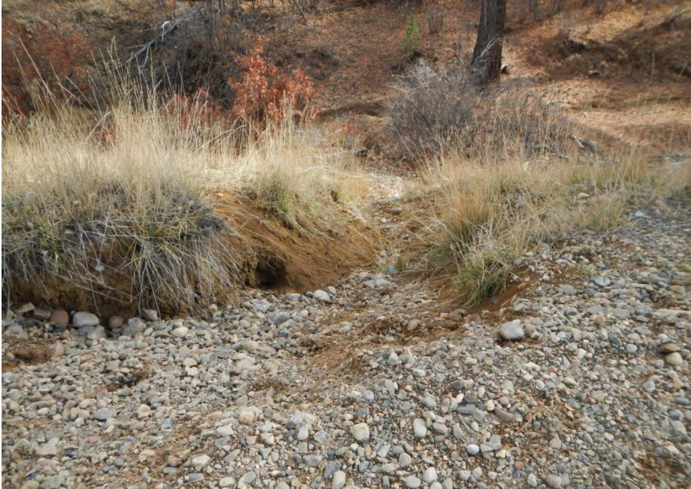
Photo 3. View of erosional channel on eastern side of access road near well pad entrance. Small amount of cobble may not be sufficient to prevent erosion here.
