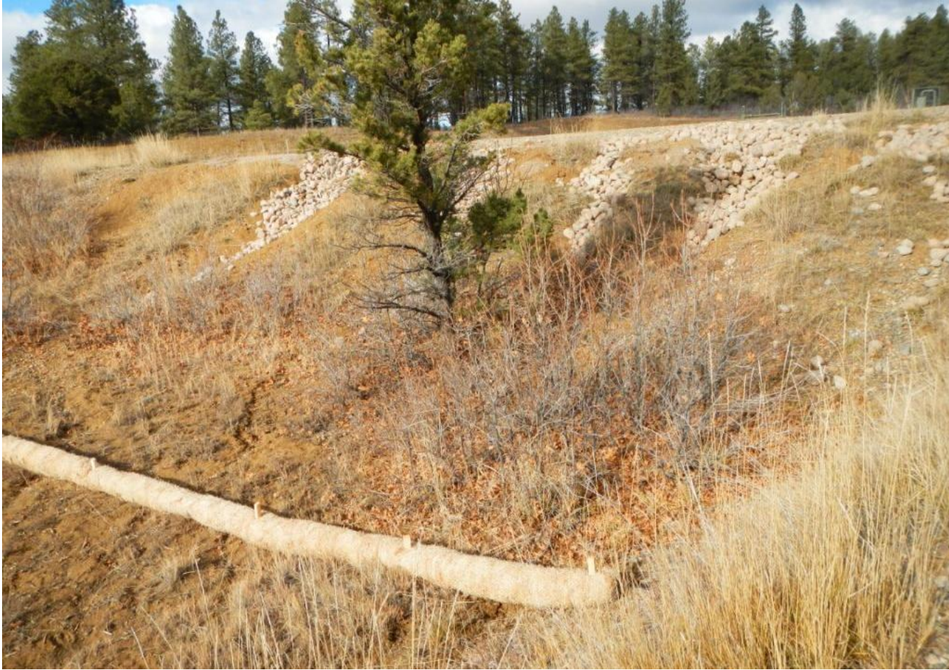
Photo 2. View of straw wattle placed below cobble in southern portion of project area.
