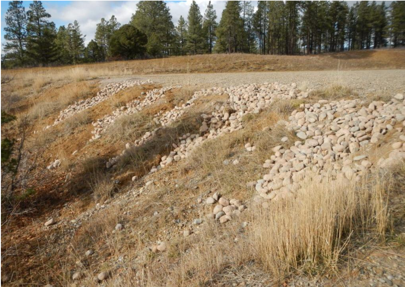
Photo 1. View of cobble placed in erosional channels in southern portion of project area.
