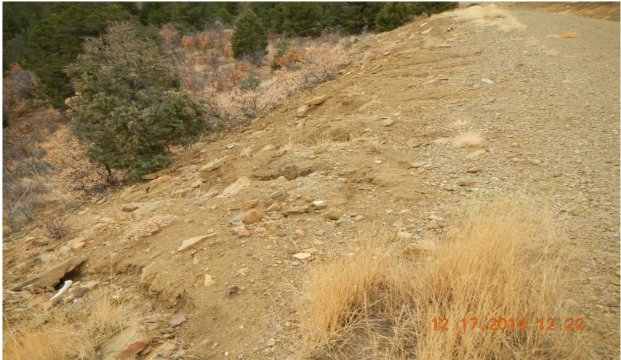
photo 5: Erosion is occurring off of the access road along the access road.
