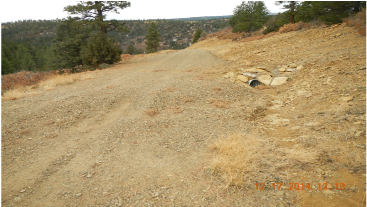
photo 3: Gravel and culverts have not been removed and the road has not been reclaimed.
