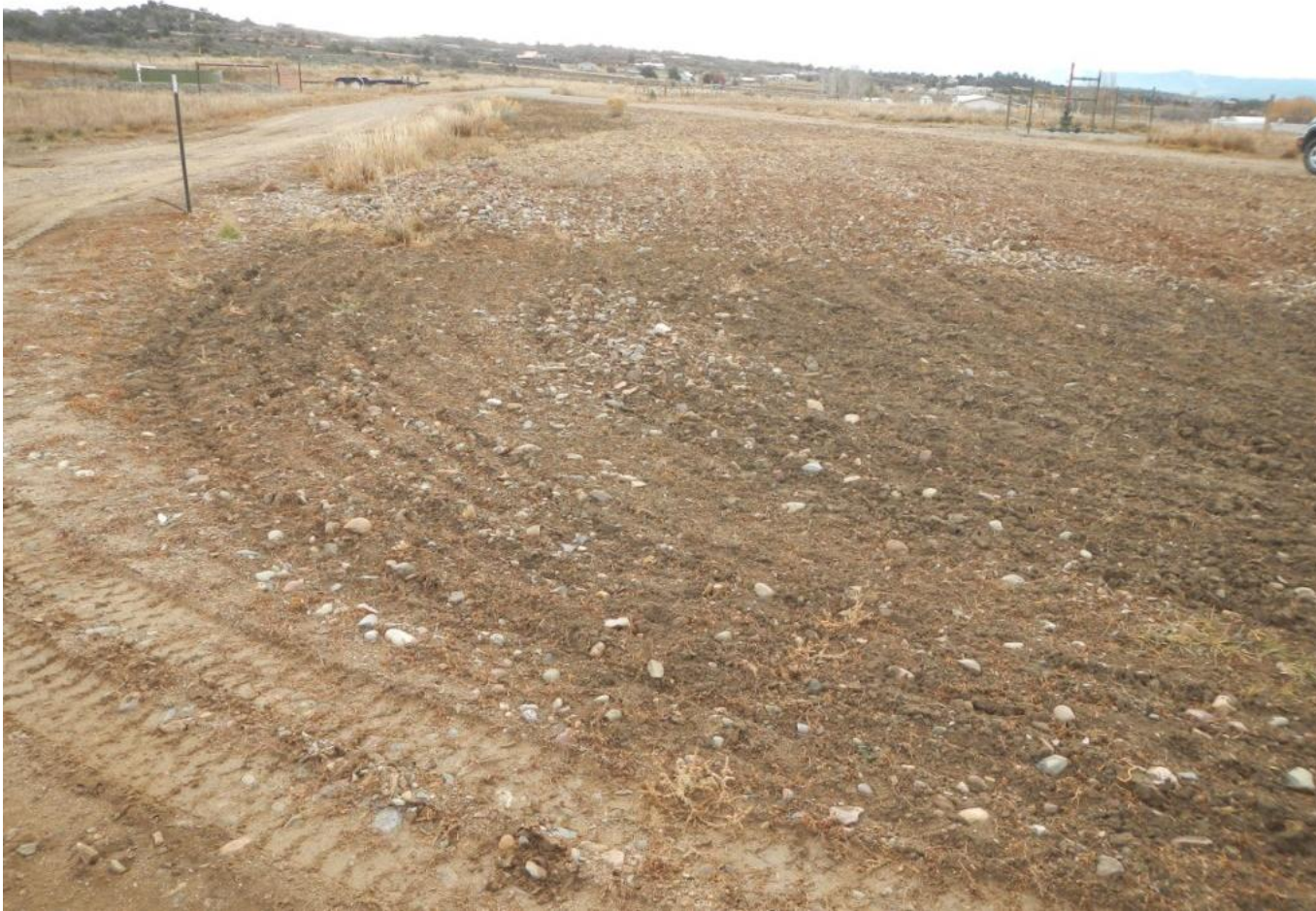
Photo 2. View of eastern portion of newly reclaimed teardrop area from northeast portion of well pad facing southward. Existing vegetation remains and Russian thistle was removed.
