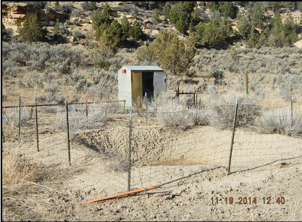
Inactive Production Pit. Weeds and vegetation. Meter house in the back looks abandoned. Broken door, broken equipment inside.
